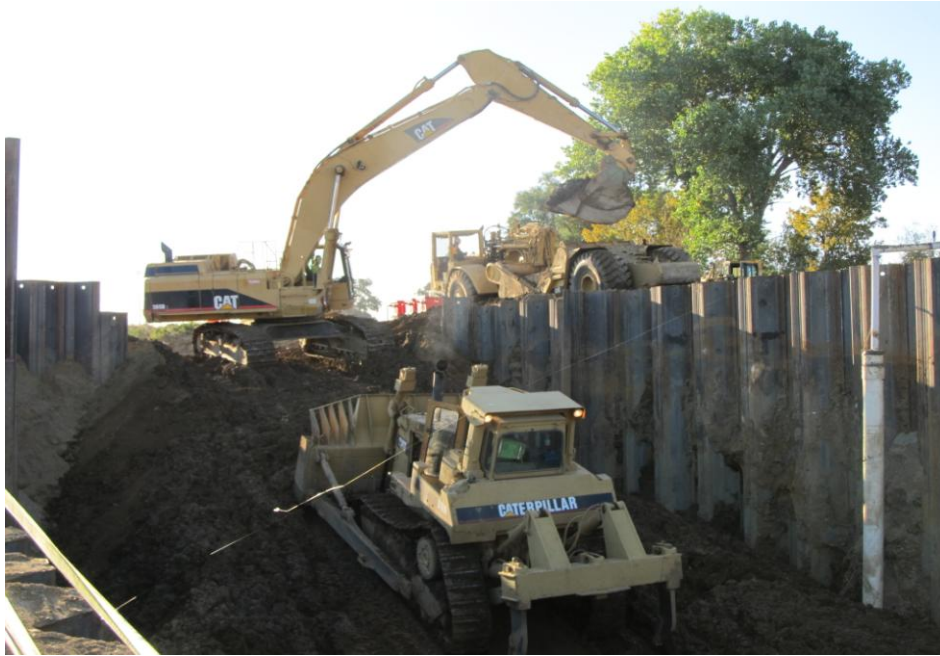
West Bay Builders Subcontractor Meyers' Dozer Pushing Material to Excavator to Load on Scraper
