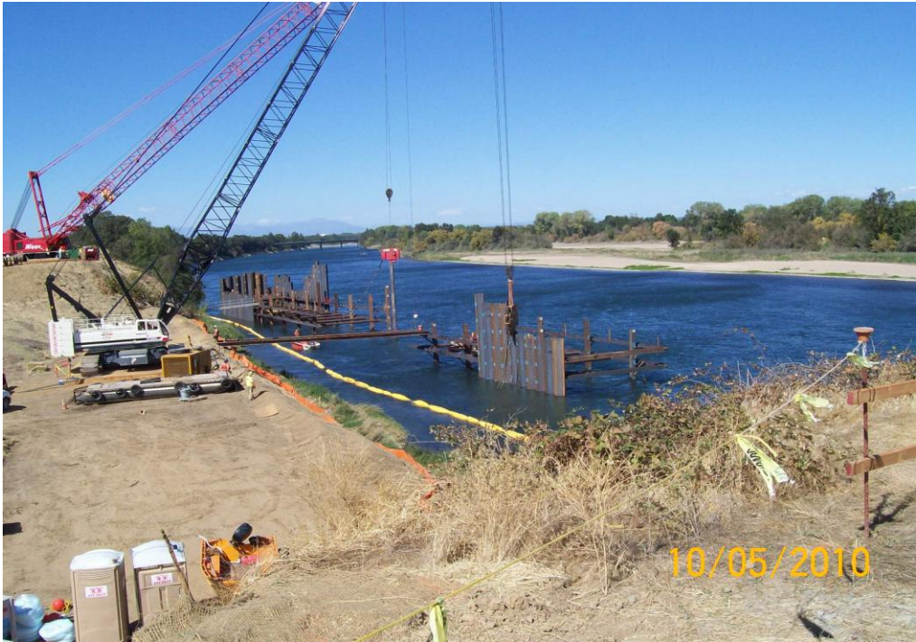
Balfour Beatty Infrastructure Installing Cofferdam Sheet Piling for Fish Screen Bay 1 to 14
