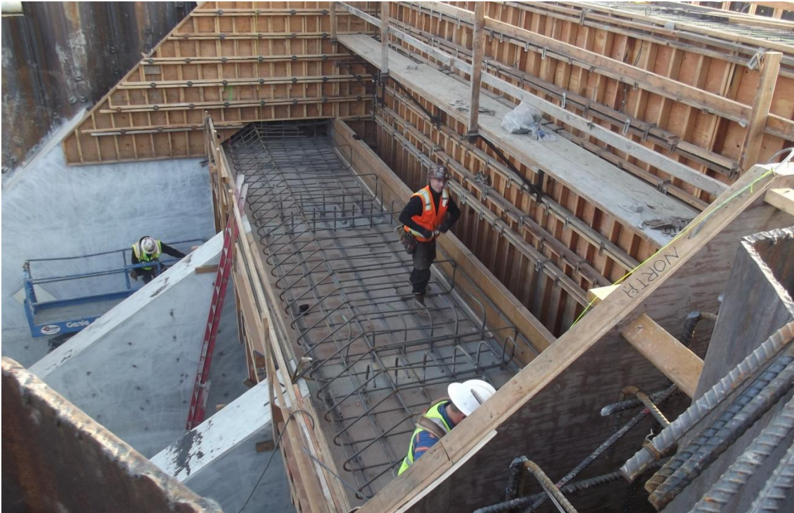
West Bay Builders subcontractor CMC Rebar installing reinforcing for the inlet structure deck.
