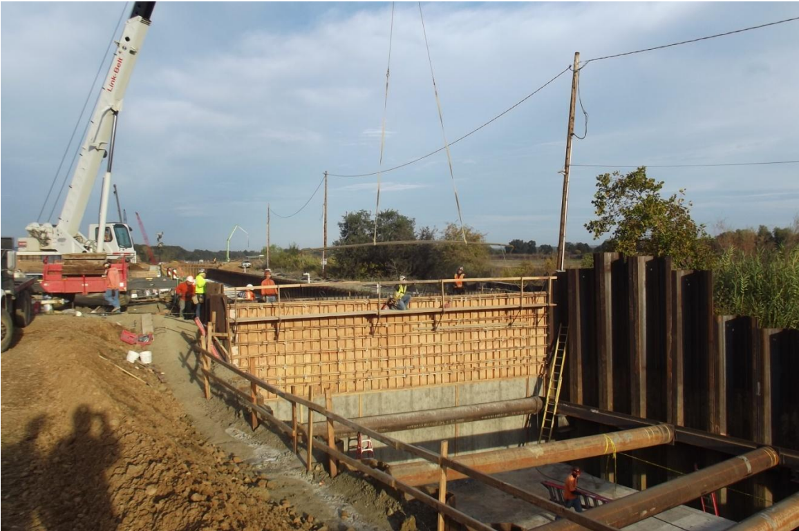
West Bay Builders carpenter crew finishing installation of forms for inlet structure.
