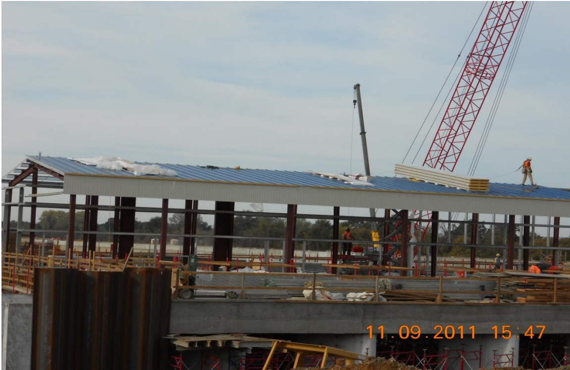
Balfour Beatty sub contractor Quality Erectors installing roof panels on Pumping Plant Control Building.
