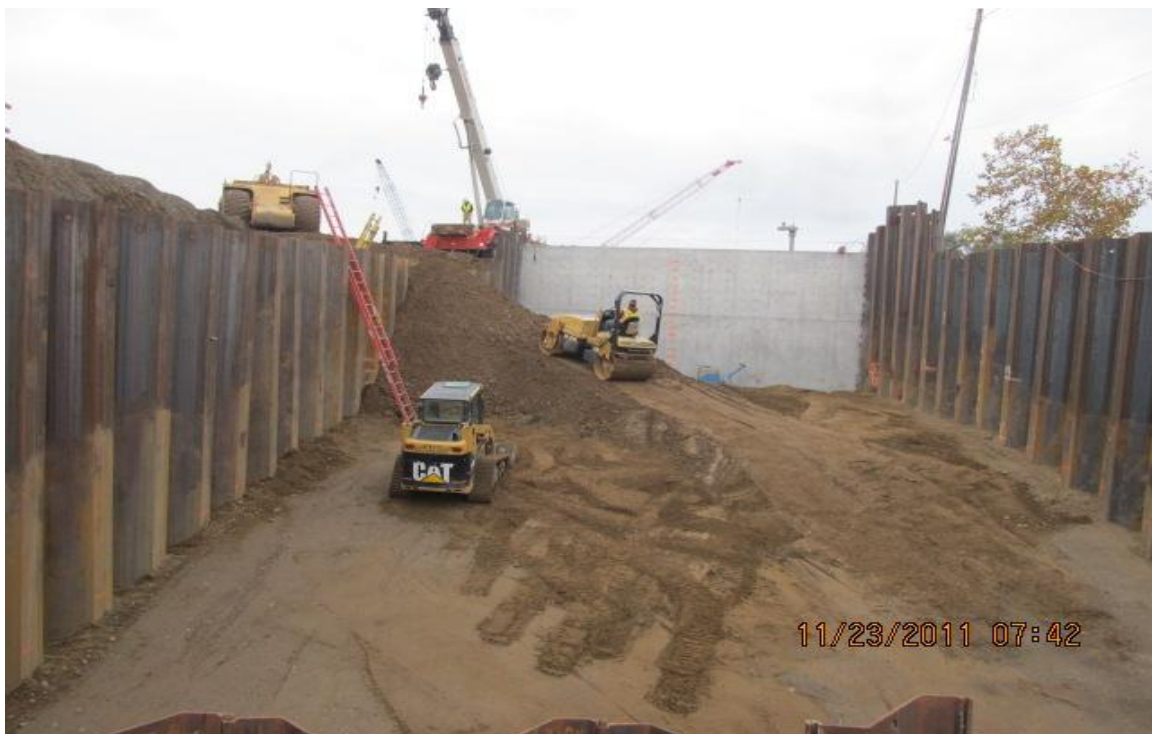
West Bay Builders subcontractor Meyers compacting backfill material to be used as an access ramp.
