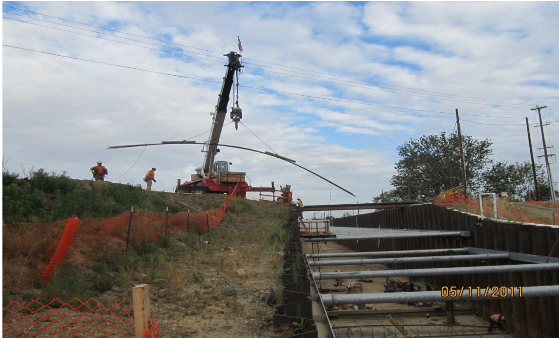
West Bay Builder's crane lowering reinforcing material for downstream canal structural concrete.
