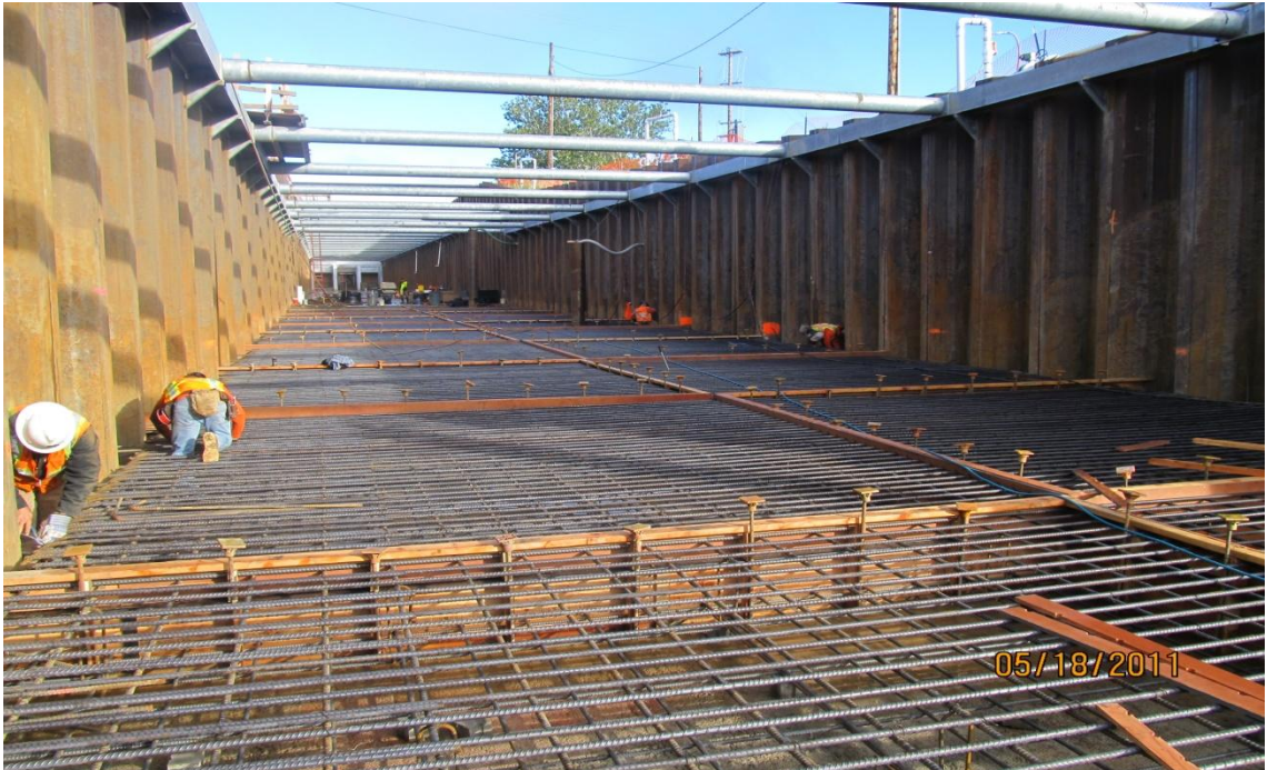
West Bay Builders subcontractor CMC Rebar installing rebar for downstream canal structural concrete.
