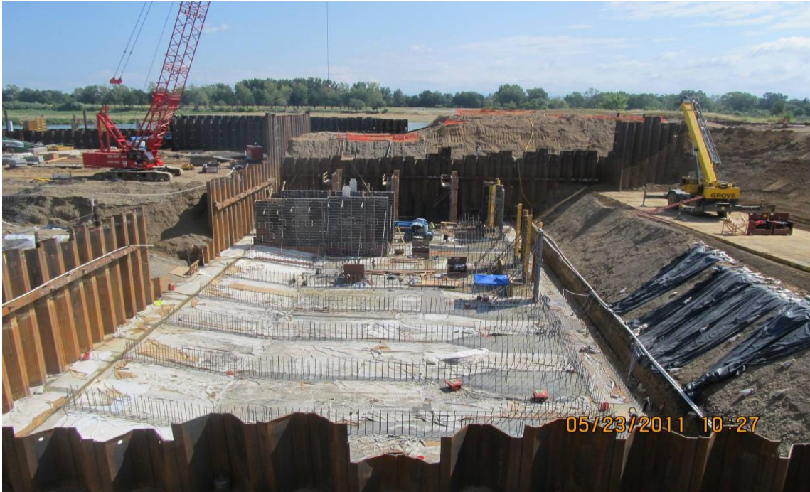
Balfour Beatty pumping plant overview, looking towards the Sacramento River.
