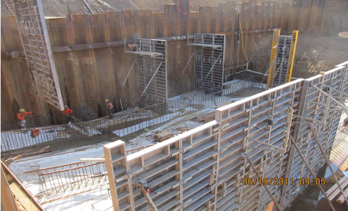
Balfour Beatty carpenters installing wall forms for the wing walls of the pumping plant.
