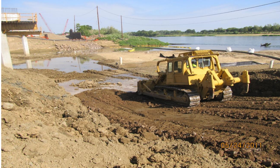
West Bay Builders subcontractor MD Site Grading building access road across Red Bank Creek.
