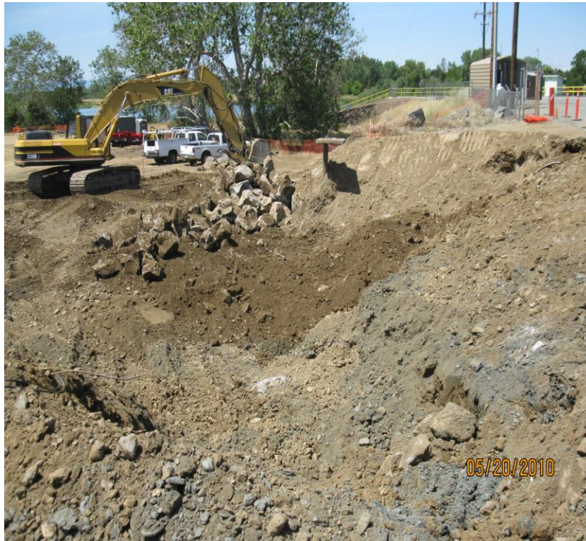
Excavating for Sheet Piles that form the Canal, east of Red Bank Creek.
