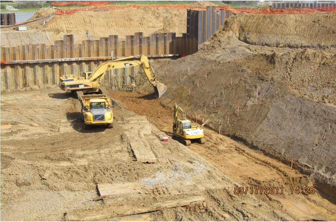
Balfour Beatty sub contractor Meyers excavating a trench near the pumping plant.
