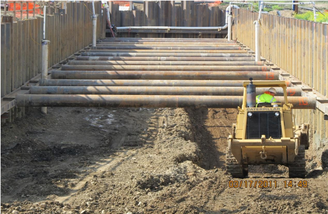
West Bay Builders subcontractor Meyers begins excavating the 2 nd lift for Phase 2 Siphon excavation.
