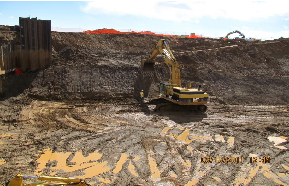
Balfour Beatty grade-checker setting grade along the slope in the pumping plant.
