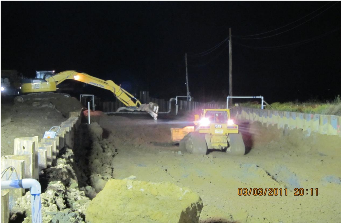
West Bay Builders subcontractor Meyers begins the Phase 2 Siphon excavation during the swing shift.
