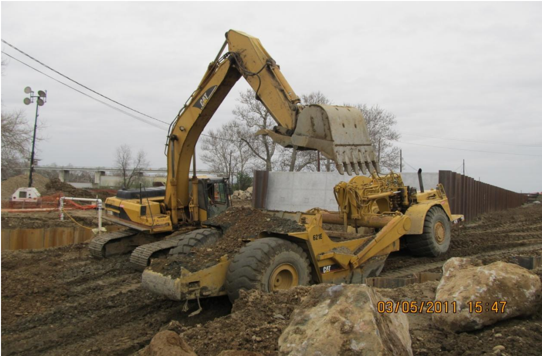
West Bay Builders subcontractor Meyers continues to remove material from the Phase 2 Siphon.
