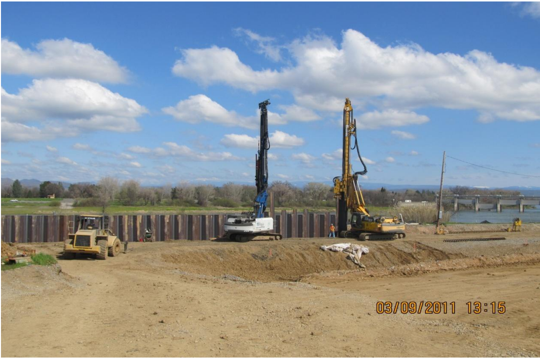
West Bay Builders subcontractor Hughes pre-drilling and driving sheet piles for the upstream canal.
