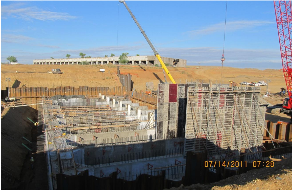
Balfour Beatty Pumping Plant overview, looking towards the forebay bank.
