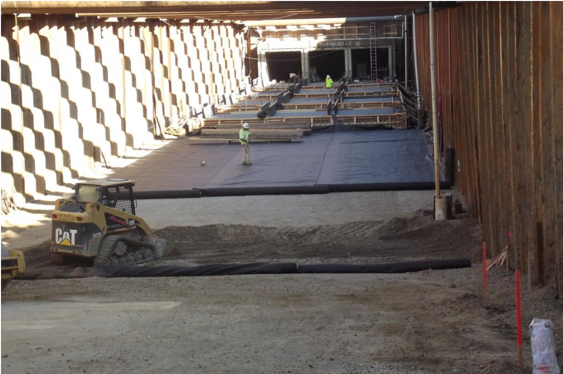
West Bay Builders subcontractor Meyers installing geo textile material over gravel fill in the Siphon.
