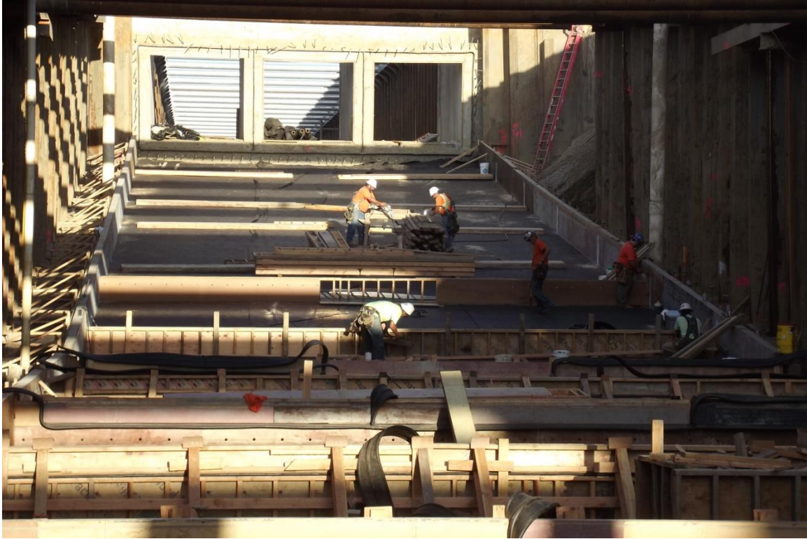
West Bay Builders carpenter crew installing formwork for Siphon Phase II concrete slab.
