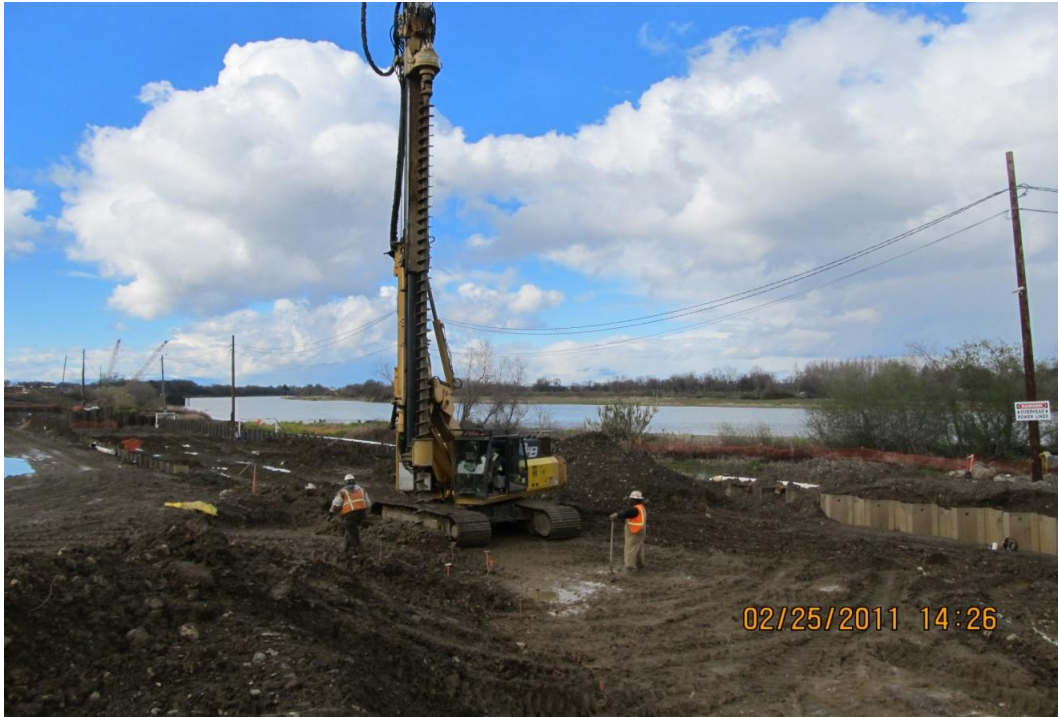
West Bay Builders subcontractor Hughes pre-drilling for pile driving Phase 2 siphon sheet pile shoring system.
