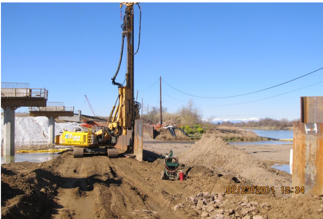
Hughes pulls temporary sheet piles for Phase 1 siphon sheet pile shoring system.
