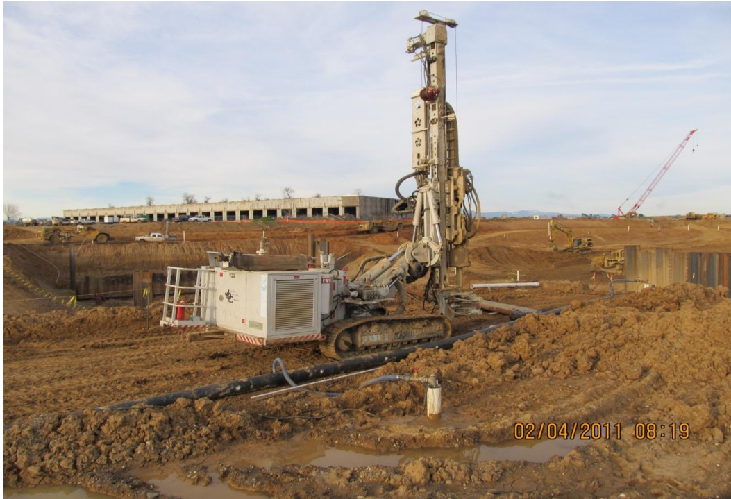
Balfour Beatty's subcontractor Jensen drilling piezometer well above the pumping excavation for dewatering.
