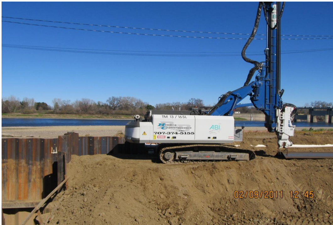
West Bay Builders subcontractor Hughes Construction driving the grade control sheet piles into place.
