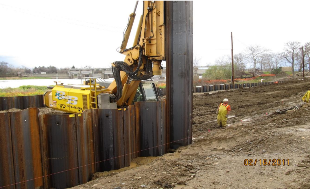
West Bay Builders subcontractor Hughes installing sheet piles on the south side of the siphon shoring Phase 2.
