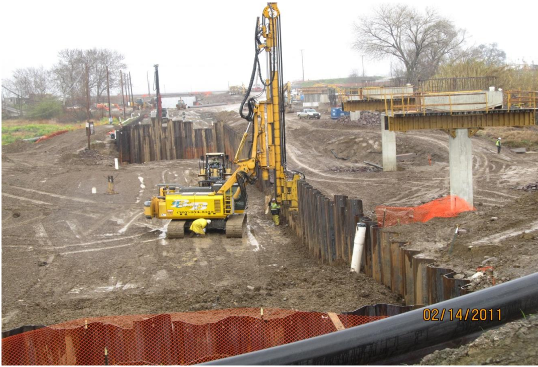
West Bay Builders subcontractor Hughes pulling sheet piles from the siphon shoring system Phase 1.
