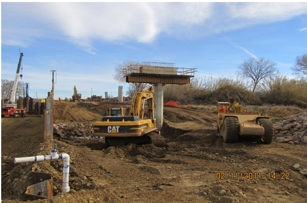
West Bay Builders subcontractor Meyers installing the siphon grade control structure in Red Bank Creek.
