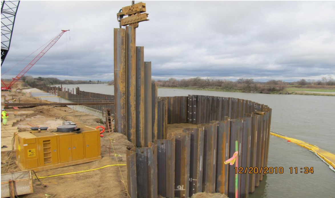
Balfour Beatty Pile Driving Downstream Forebay and Fish Screen Sheet Pile Wall
