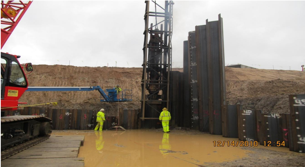
Balfour Beatty's Diesel Pile Driving Hammer Driving Sheet Piling on Pumping Plant Wall
