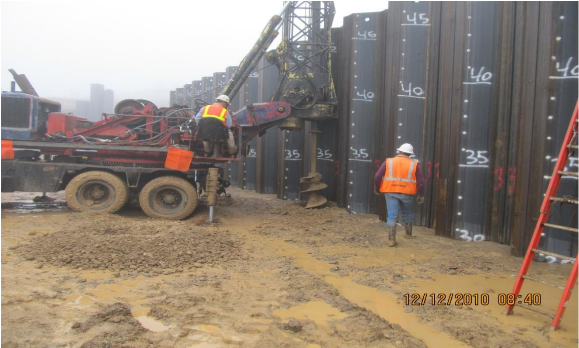
Balfour Beatty Subcontractor Jensen Drilling, Drilling Inside Pumping Plant Sheet Pile Wall to Help Reduce Driving Pressure
