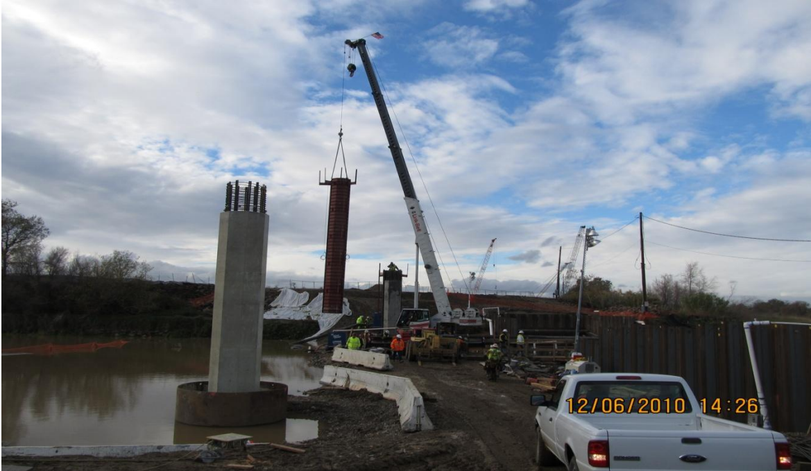
West Bay Builder's 50 TN Link Belt Crane Stripping the Forms Off Bridge Column
