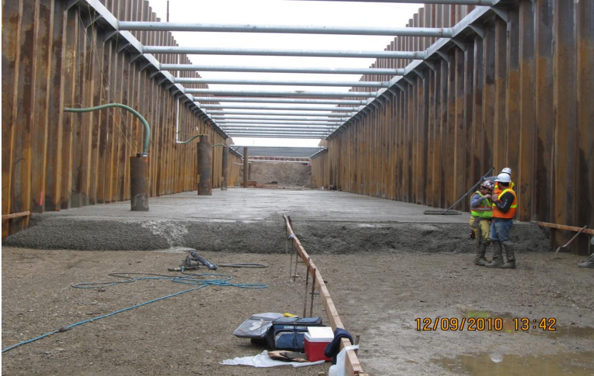
West Bay Builders Subcontractor Landavasso Brothers Placing the Downstream Canal Lean Concrete Slab on Grade
