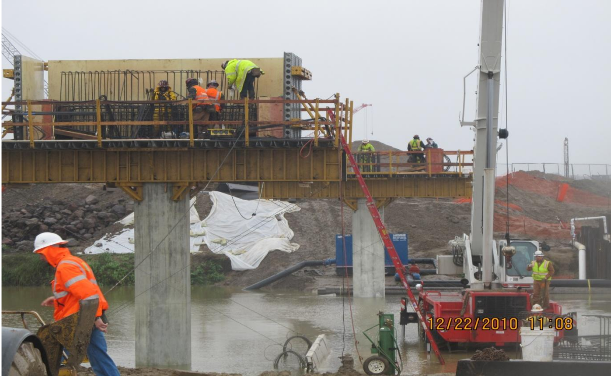
West Bay Builders Formwork and Rebar Installation on Bridge Columns #2 and #3 in Progress
