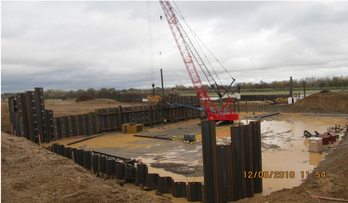
Balfour Beatty Driving of Upstream Face of Pumping Plant Sheet Pile Wall
