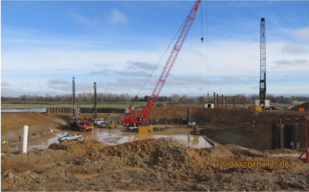
Balfour Beatty's Subcontractor Jensen Drilling Drilling Relief Holes Along the Pumping Plant Forebay Sheet Pile Wall
