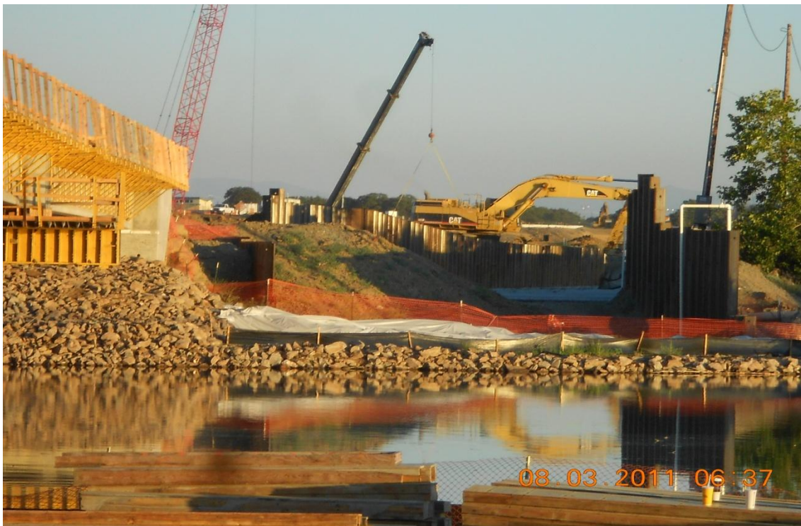
West Bay Builders subcontractor Meyers using excavator to dig out upstream canal.
