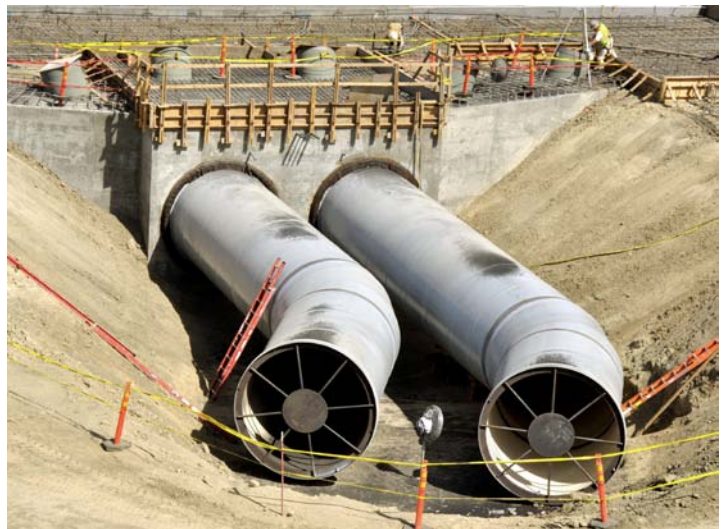
Constructing the Intertie pipes that connect the Delta-Mendota Canal to the California Aqueduct.
