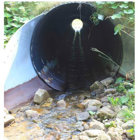
This culvert on Oats Run in Pocahontas County, WV had been blocking brook trout from moving throughout their historic range.
