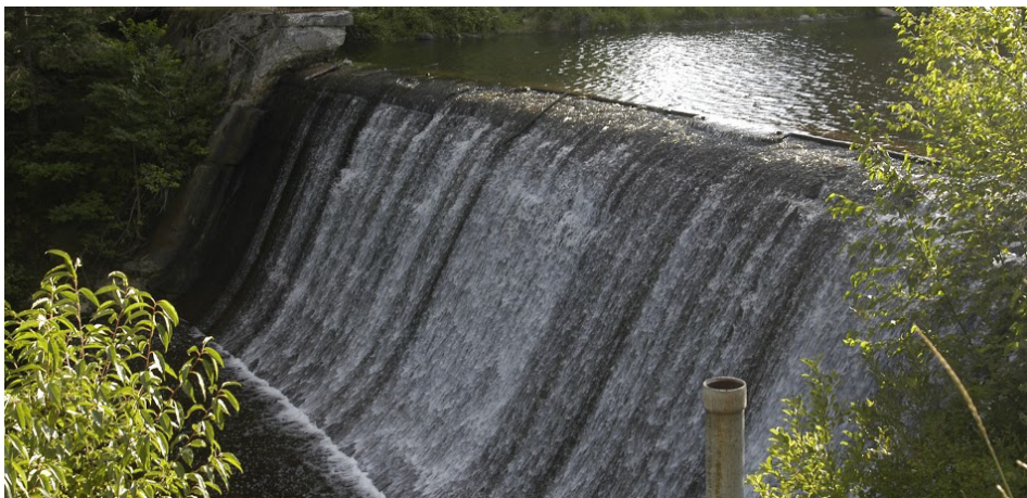
Small dams like this one on the Chubb River in NY block fish migration, can be dangerous to people and during flooding, represent a potential hazard to downstream property.
