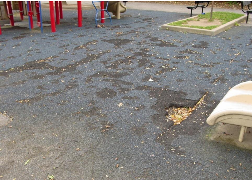
BEFORE - After capping it for the 2nd time, PIP systems is simply not strong enough
