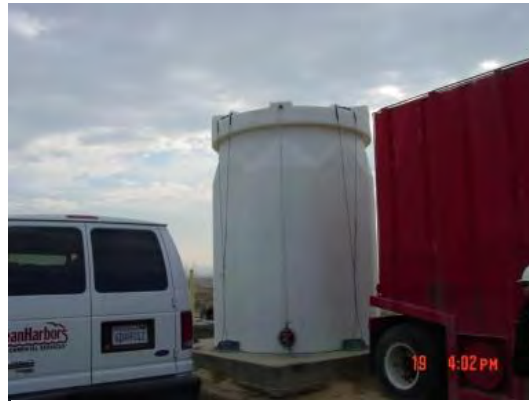
Sony DSC-S75, Photo #11; View of a 5,000-gallon, white plastic, leachate collection tank at WMU 35 Cell #3, facing west.
