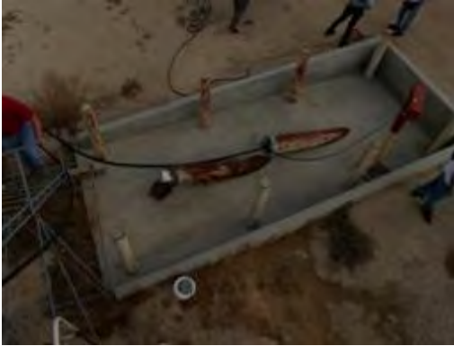
Olympus Stylus 8000, Photo #76; View of the leachate collection system at WMU 28 from the top of the leachate collection frac tank (Frac Tank 3).
