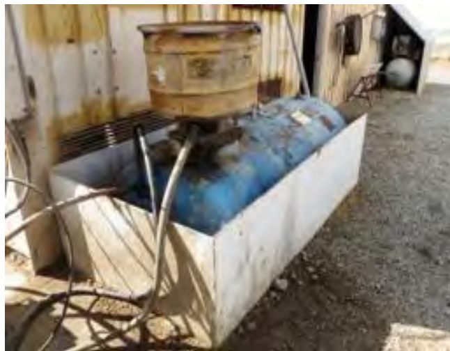
Olympus Stylus 8000, Photo # 50; View of the used oil storage tank at the maintenance building.
