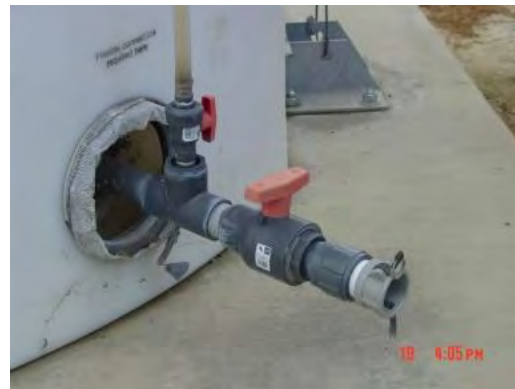
Sony DSC-S75, Photo #12; View of the piping and valve for draining the 5,000-gallon, plastic, leachate collection tank at WMU 35, Cell #3, facing northwest. Note: no secondary containment or cap/plug.
