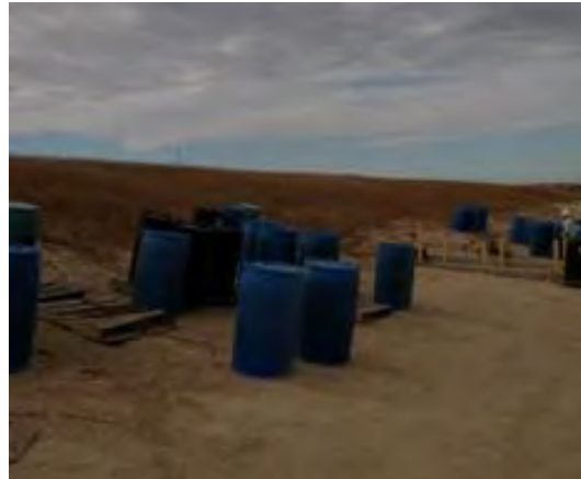
Olympus Stylus 8000, Photo #82; View of the leachate collection system and less-than-90-day storage area at WMU 33 Cell #3B.
