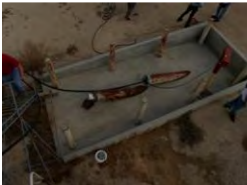
Olympus Stylus 8000, Photo #76; View of the leachate collection system at WMU 28 from the top of the leachate collection frac tank (Frac Tank 3)
