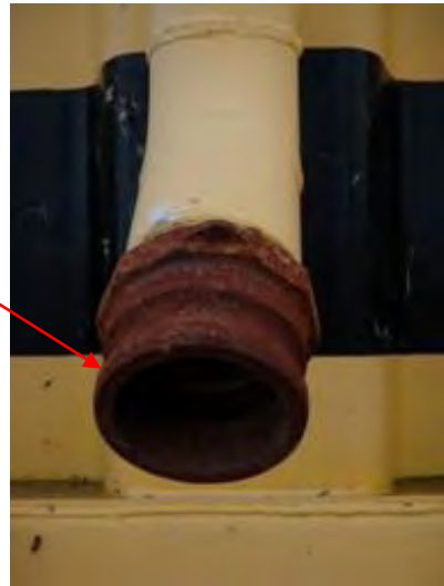
Olympus Stylus 8000, Photo #99; View of the open pumping port at the rear of the leachate collection frac tank (Tank 80) at WMU 35, Cell #1.
