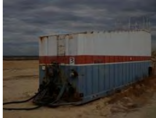
Olympus Stylus 8000, Photo #73; View of the leachate collection frac tank (Frac Tank 3) at WMU 28.
