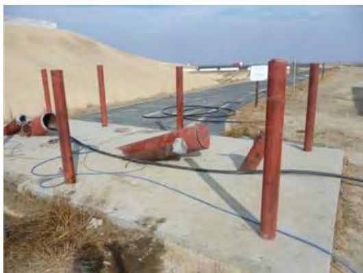
Panasonic Lumix DMC-TZ5, Photo #17; WMU 34 leachate collection ports, facing northeast.
