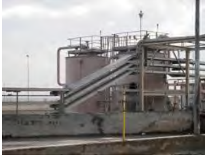
Olympus Stylus 8000, Photo #6; View of the RCRA-permitted water (left) and dirty water (right) storage tanks, facing southeast.
