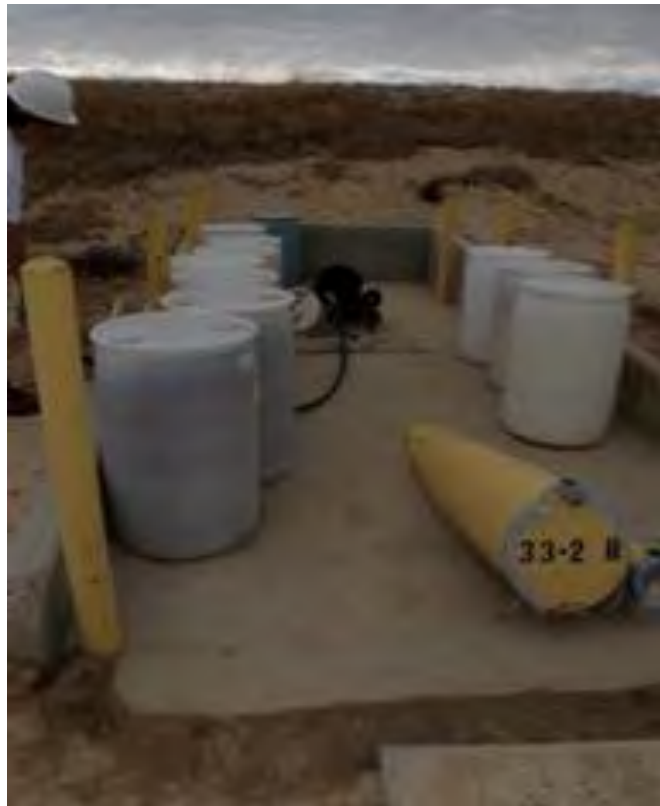
Olympus Stylus 8000, Photo #90; View of the leachate collection system at WMU 33, Cell #2. One, full 55-gallon container of F039 leachate, dated 10/13/10 to the left.
