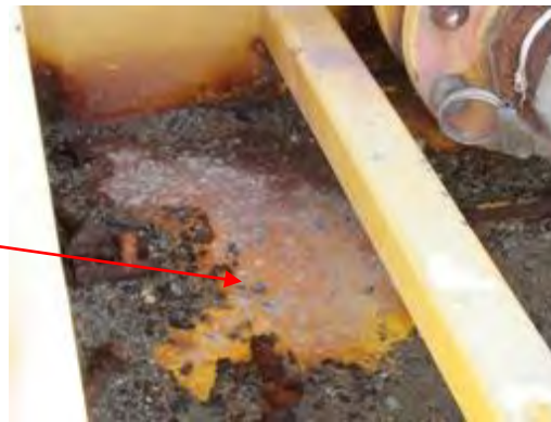
Olympus Stylus 8000, Photo #57; Close-up view of the ground near the valve of the leachate collection frac tank at WMU 34. Note the visible staining.
