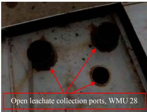
Olympus Stylus 8000, Photo #74; View of top of the leachate collection frac tank (Frac Tank 3) at WMU 28. Note the open ports.
