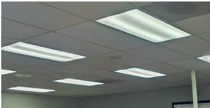
City Hall Main Office Lighting
