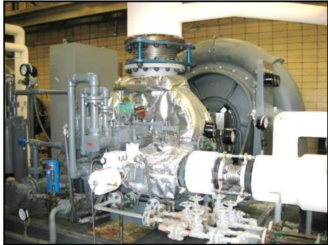
Rehabilitated Blowers equipped with Steam-Turbine Drives
