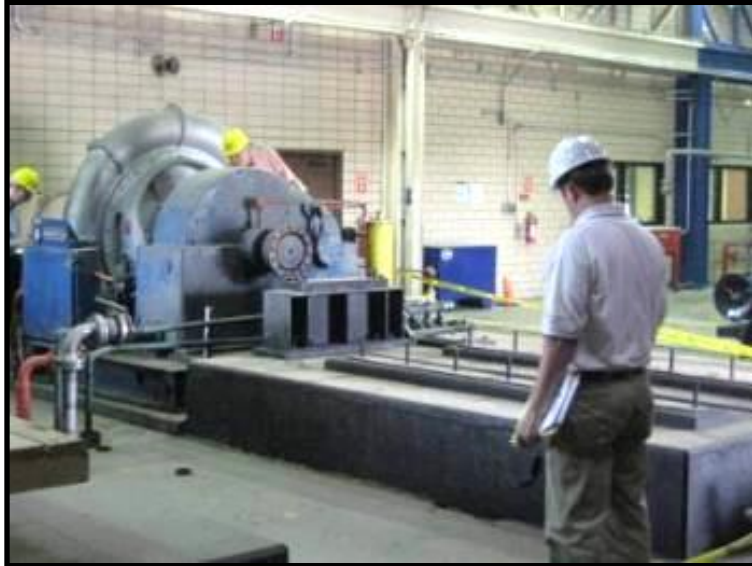
2-unused, 1,200-HP 31,000-cfm Blowers
