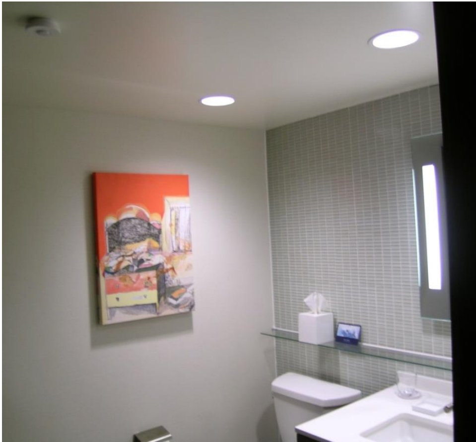
Figure 8: Bathroom downlighting (PNNL photo)
