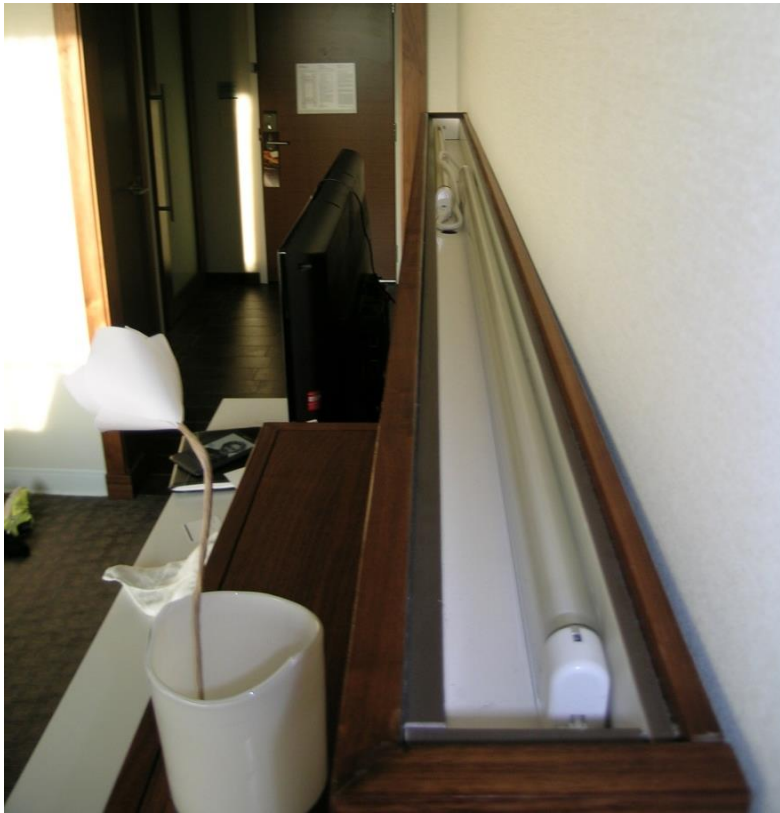
Figure 10: Millwork fixture behind television, with lens removed (PNNL photo)
