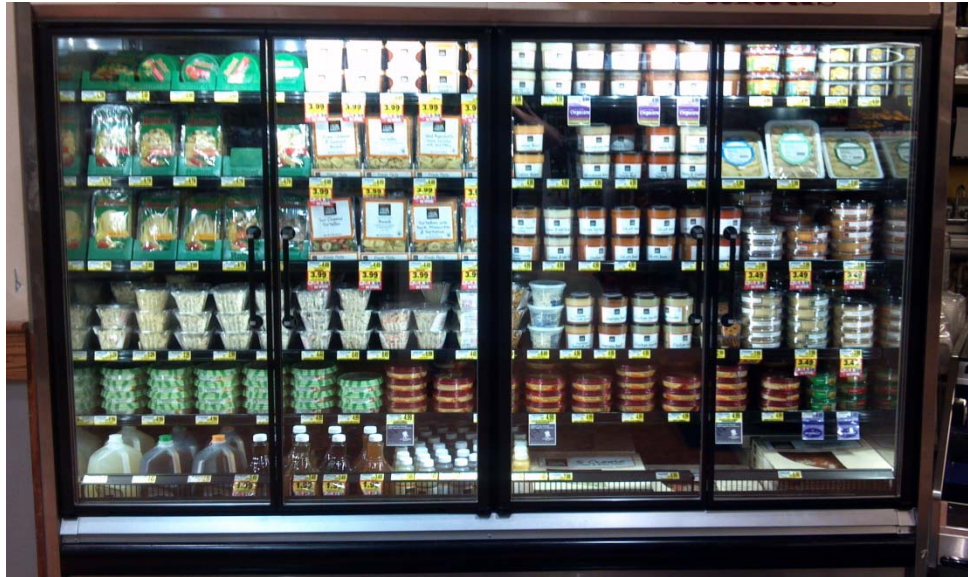
Figure 10: Example of finished display with retrofit doors in place
