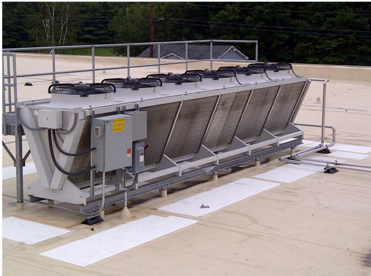
Figure III-4 Rooftop Gas Cooler
