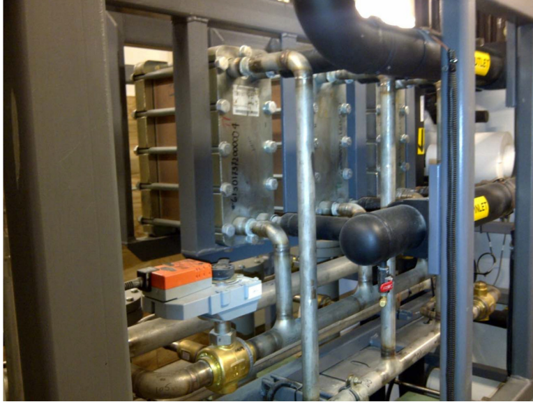
Figure III-3 High Burst Pressure Stainless Steel Piping
