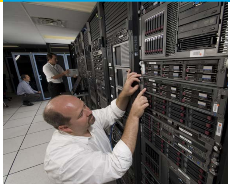
Figure 1. NREL's legacy data center
