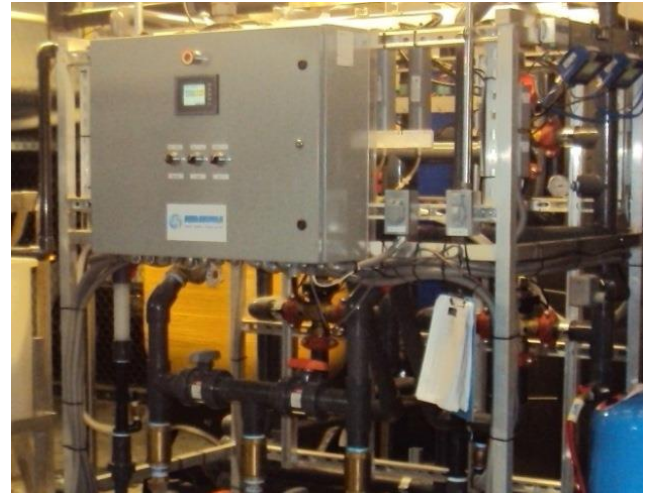
Wastewater recycling system control panel
