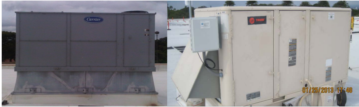
Figure 5. (a) One of the four 30-ton Carrier RTUs (left) and (b) one of the five Trane RTUs (right)
