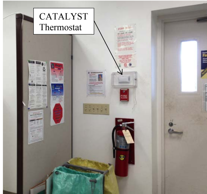
Figure 22. Building C27 improperly located temperature sensor immediately next to the side exit door
