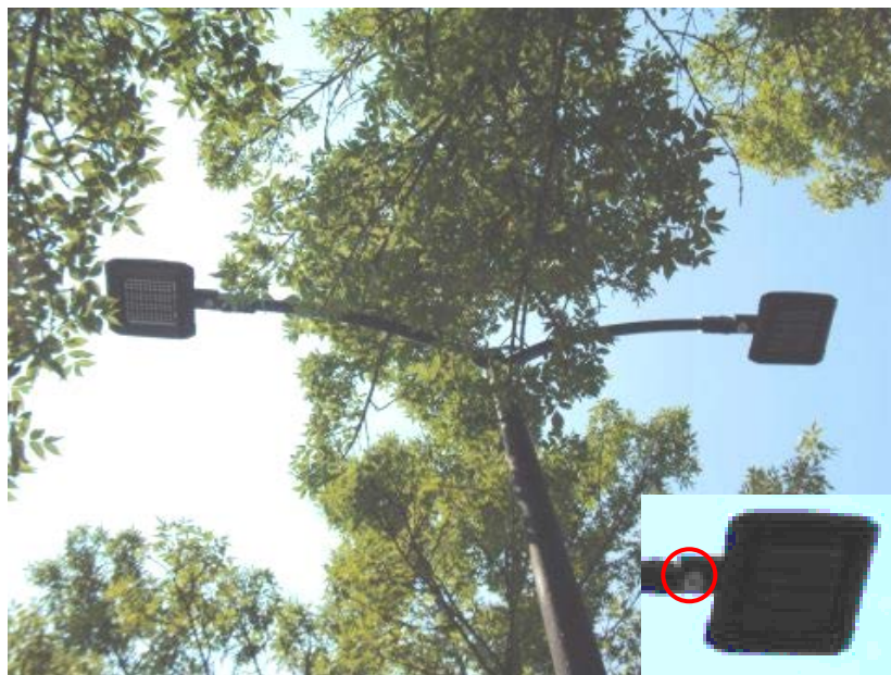
Figure 3.5. Replacement LED luminaires on extended arms and inset highlighting occupancy sensor
