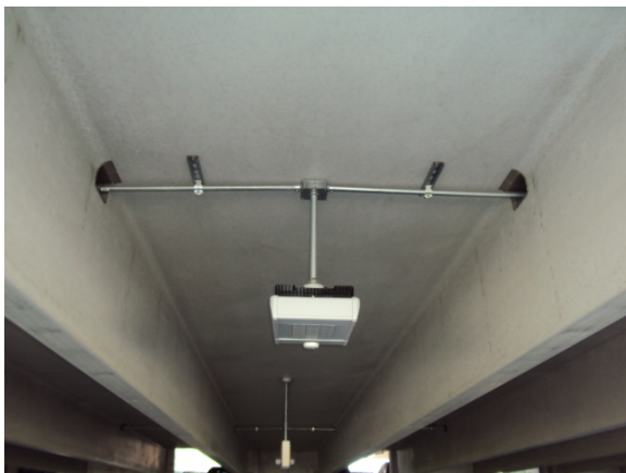
Figure 2.8. LED luminaire and pendant installation
