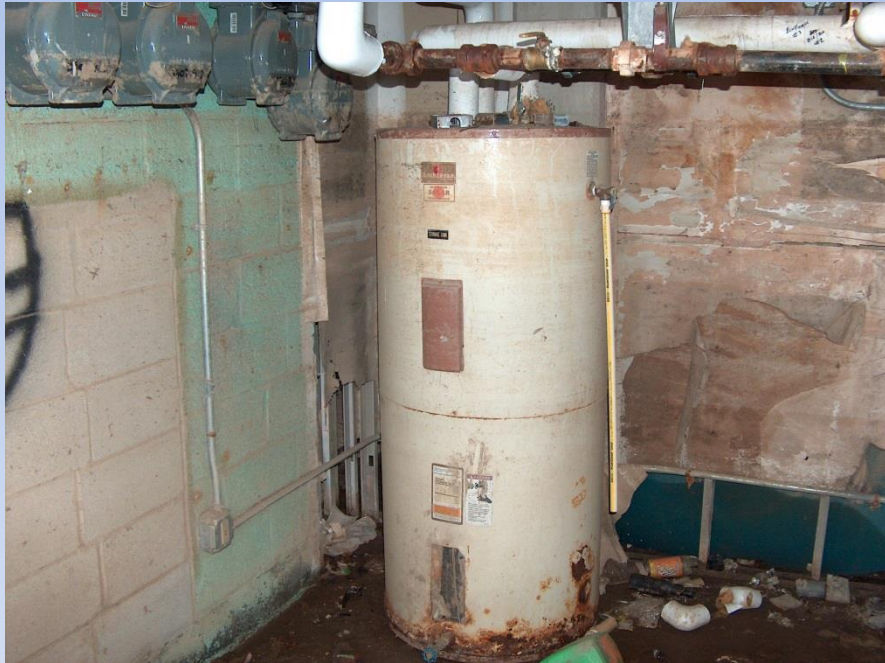
CH H 2 O Heater/Gas Submeters
