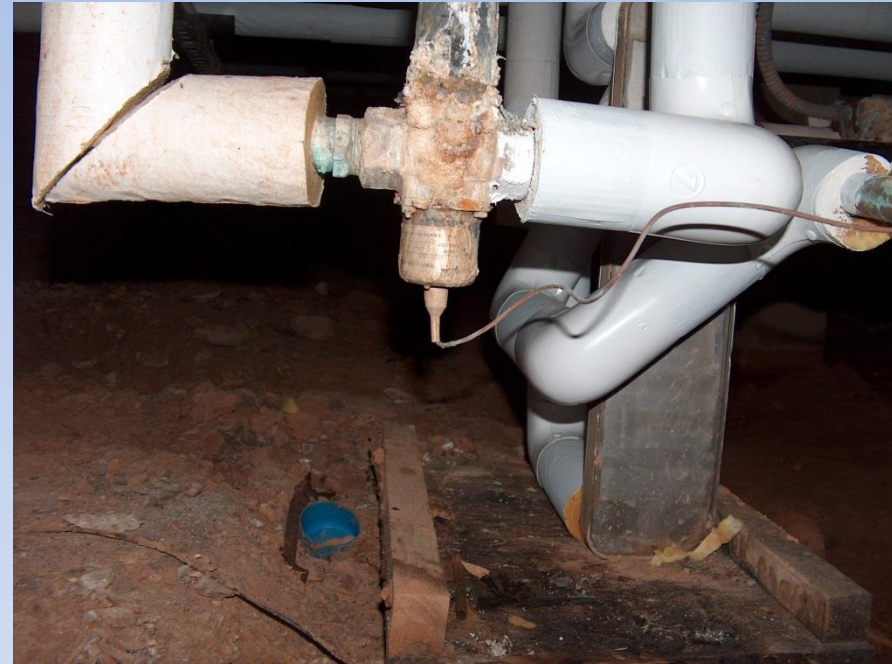
DHW Control Valve
