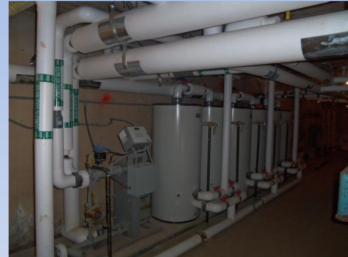
Latrobe DHW System
