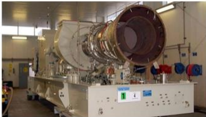
Photo: The U's Cogeneration Turbine & Generator
