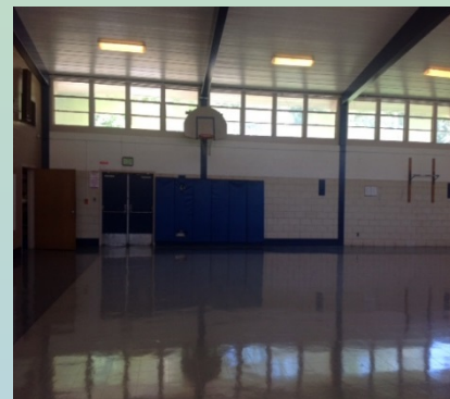
Gym Lights Before Retrofit
