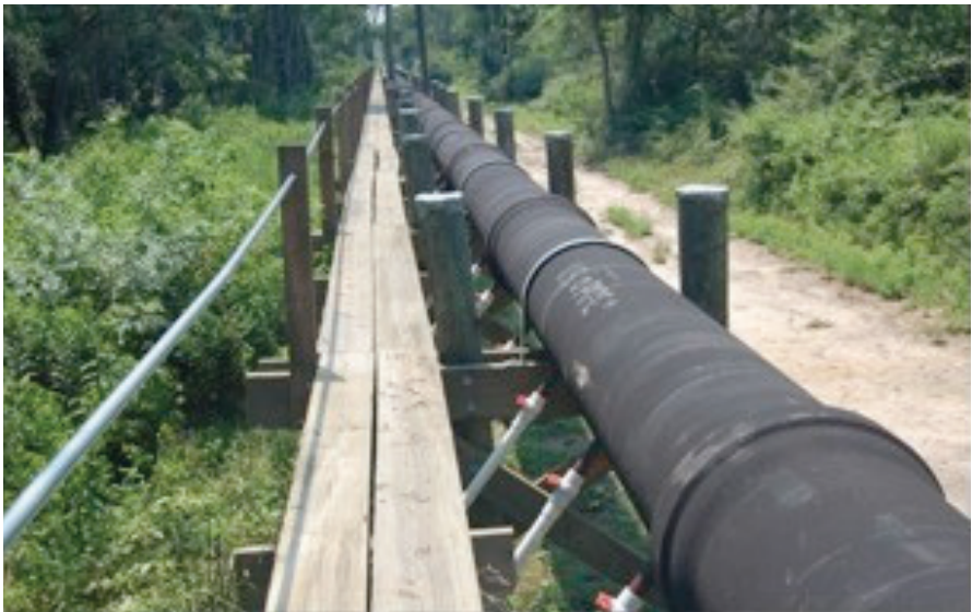
Figure III-6. Distribution pipe system for effluent at the Hammond Wastewater Treatment Plant along South Slough wetland (photo: T. Scott, 2007).
