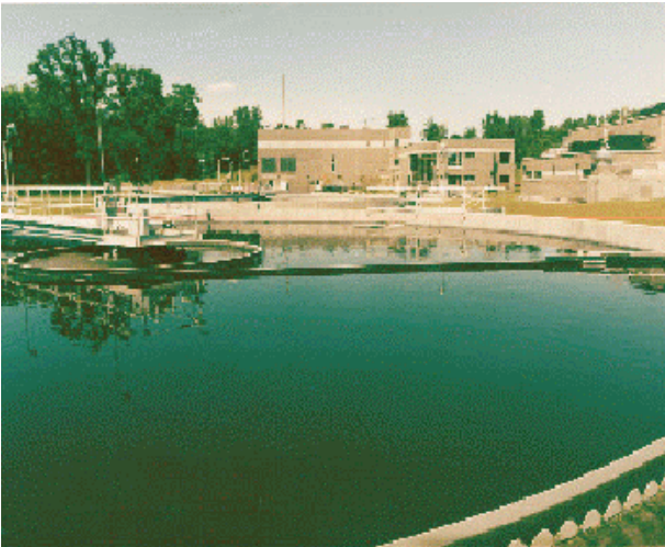
Figure I-3: Photograph of a secondary clarifier in a wastewater treatment system. ( http://www.rpi.edu/dept/chem-eng/BiotechEnviron/TreatmentPlants/GlensFalls/clarify.html )
