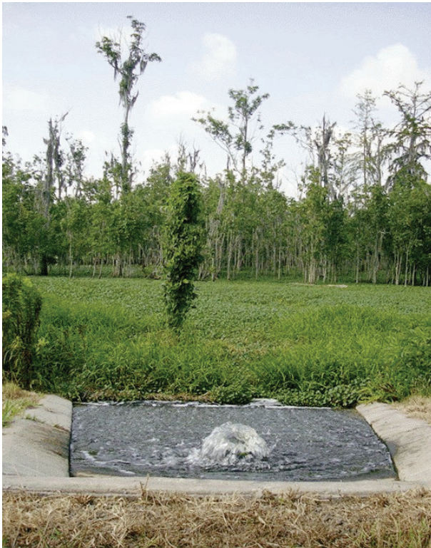
Figure III-2. Effluent distribution pipe for Thibodaux treatment plant at Pointe-au-Chene Swamp. ( www.comiterecrouces.net )
