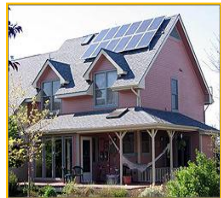
Figure 14: Photovoltaic solar panels installed on the roof of a home in Boulder, Colorado Source: NREL.gov
