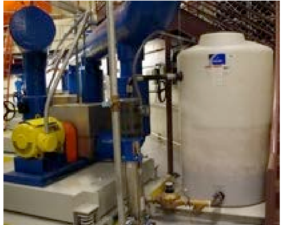
Condensate Capture System
