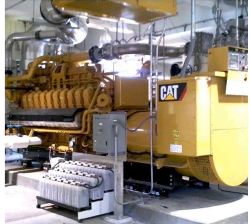
Combined heat & power system 1.6-MW engine
