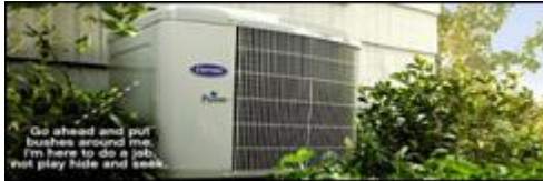
Heating, ventilating, cooling & refrigeration systems
