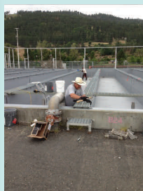
Staff put the finishing touches on the SCS raceways
