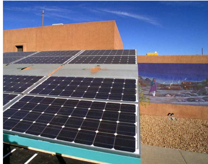
At the Indian Pueblo Cultural Center in Albuquerque, New Mexico, this photovoltaic carport delivers about 23 megawatt-hours of clean electricity to the local utility grid. Photo from Sandia National Laboratories, NREL 08978
