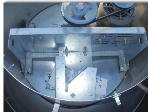
Exhaust fan with hinged base – exhaust fan screwed down, hinged base still inside
