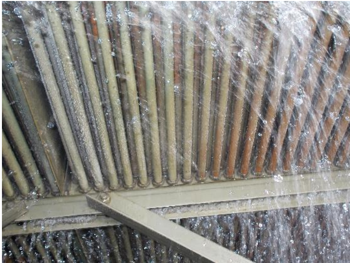
Scale forming on tubes in evaporative condenser
