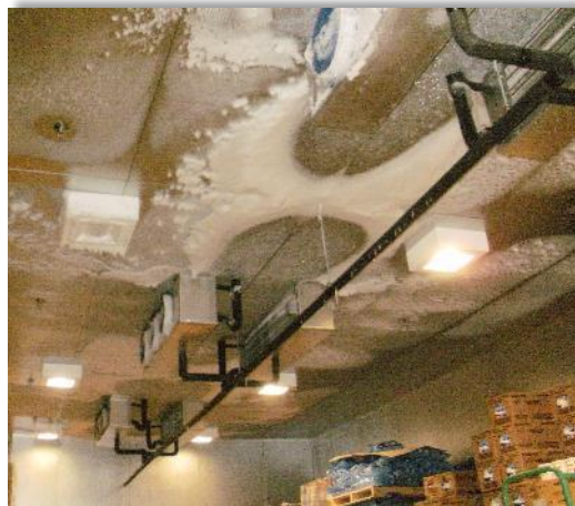
Walk-in Freezer not defrosting properly; frost buildup on ceiling
