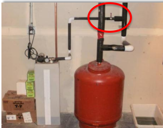
Glycol feeder is empty and valved-off
