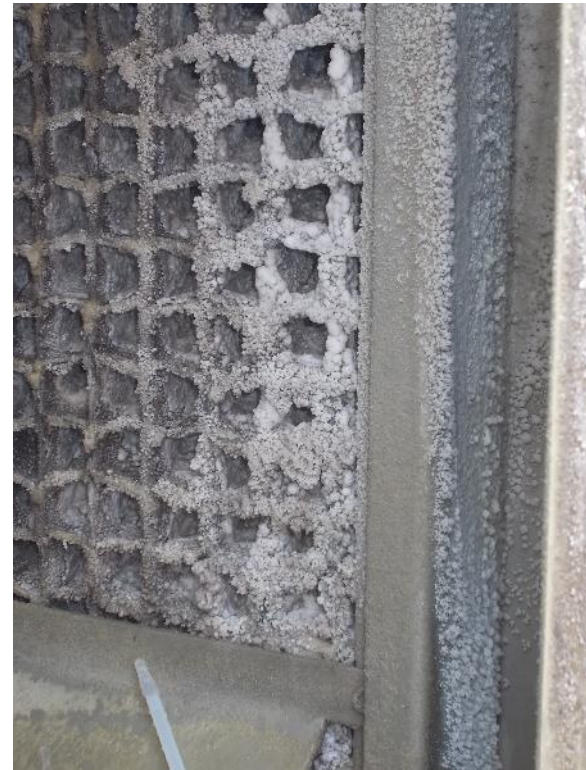
Scale forming on water tower inlet air splash screens
