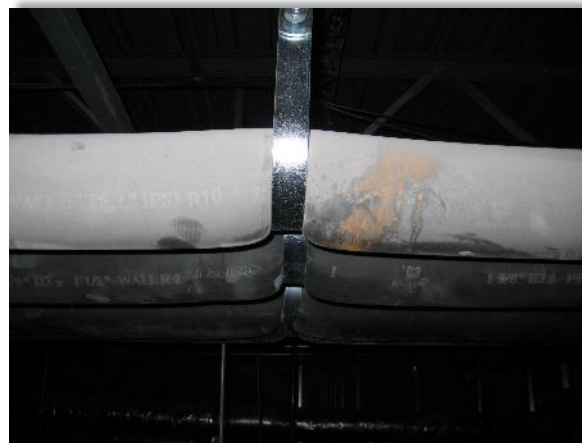
Improperly supported refrigeration piping
