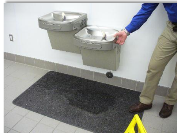
Water from drinking fountain running onto floor
