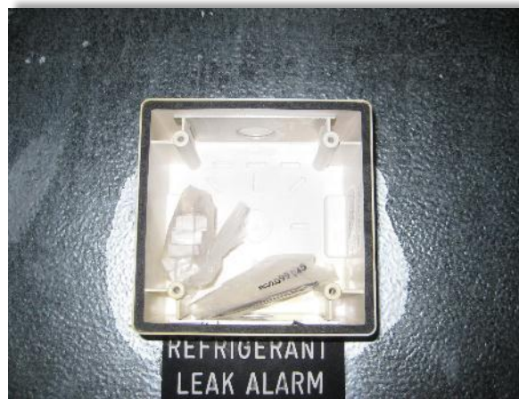
Interior of refrigerant leak detection alarm box NOTE: No control conductors
