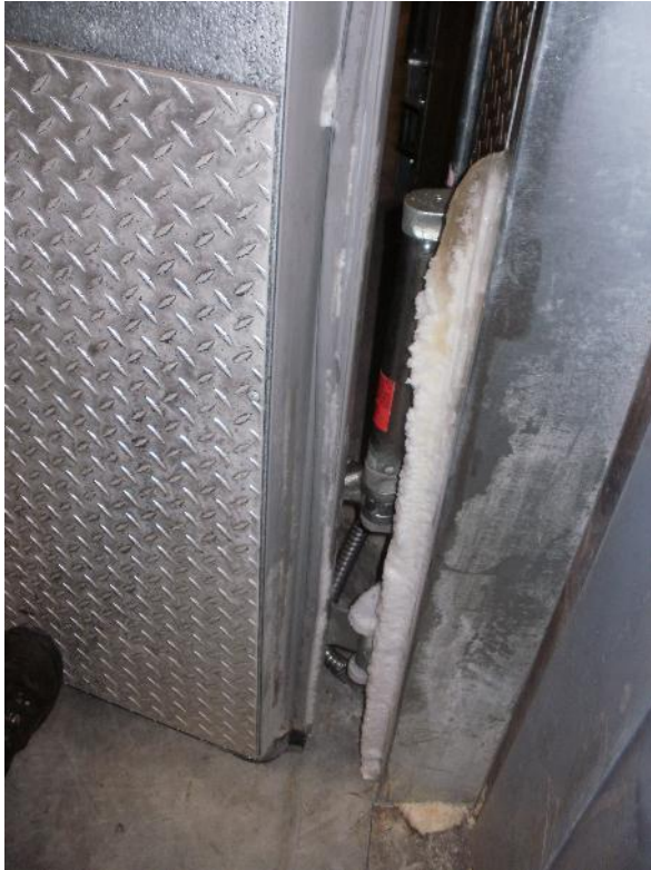
Walk-in Freezer door heater not working properly
