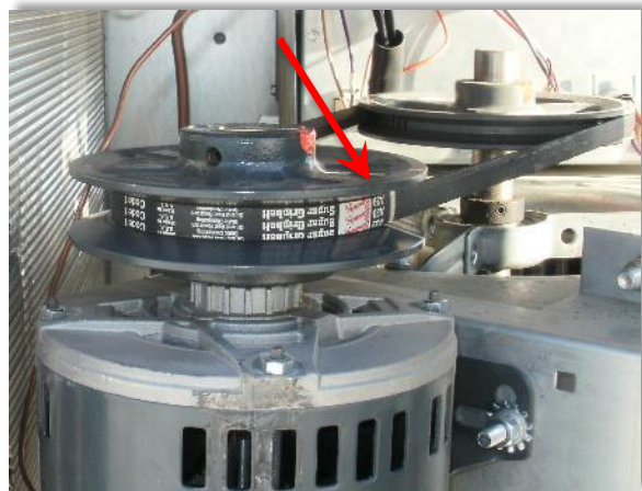
Belt out of alignment
