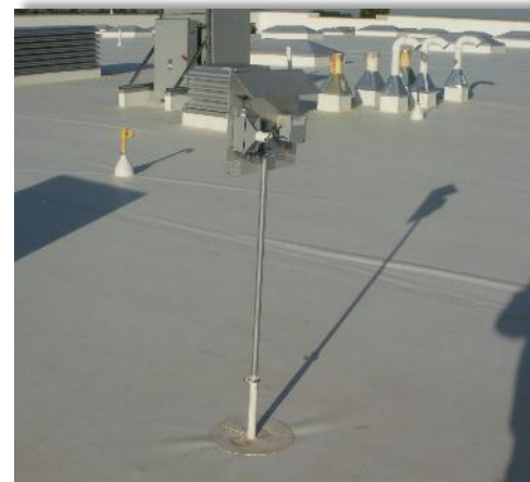
Outdoor weather station mounted in direct sunlight
