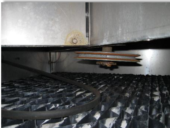
Thrown drive belt and worn bearing
