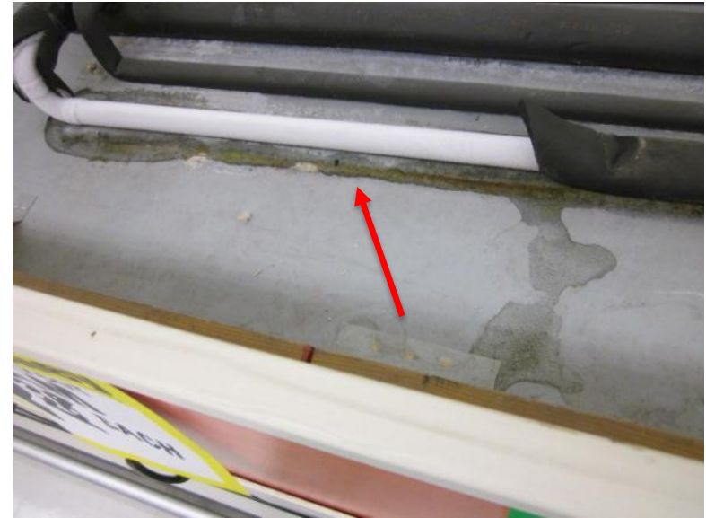
Missing insulation on top of glass door case; water is pooling and running towards the front of the case and down the door frame
