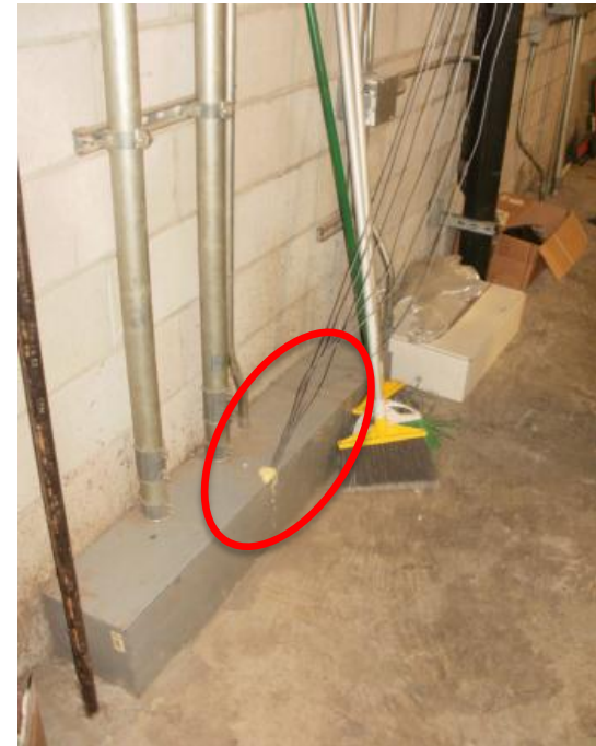
Refrigeration control wires improperly mounted
