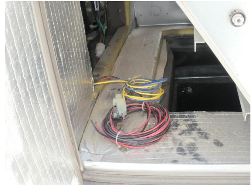
Economizer coiled up and in factory tie wraps; not hooked up
