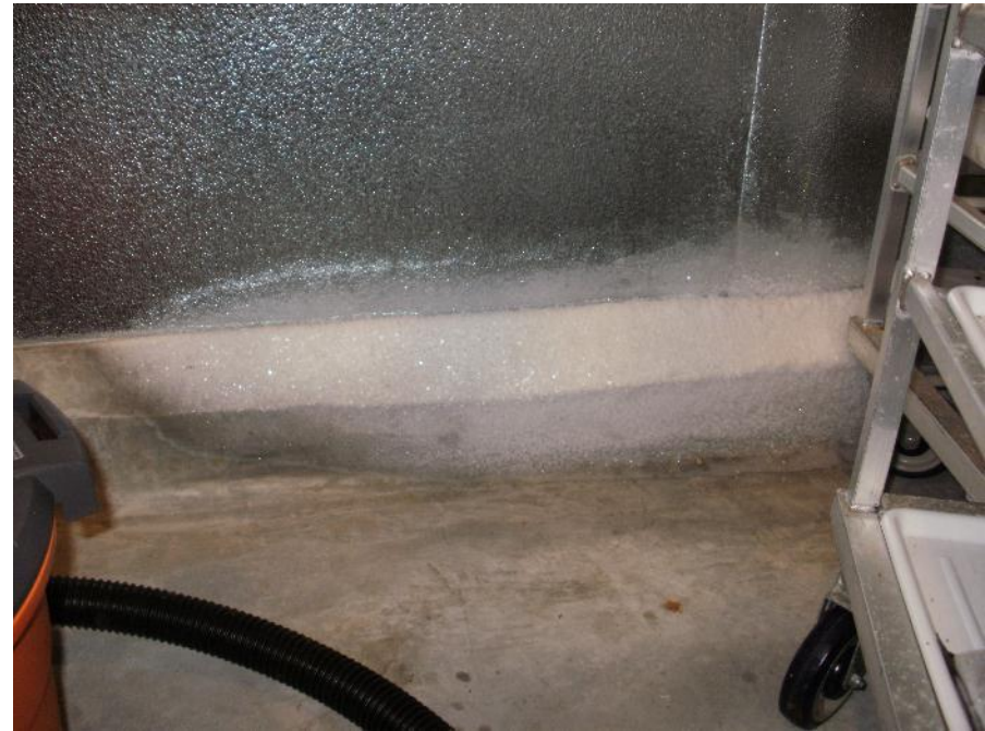
Ice building up on curb of walk-in freezer
