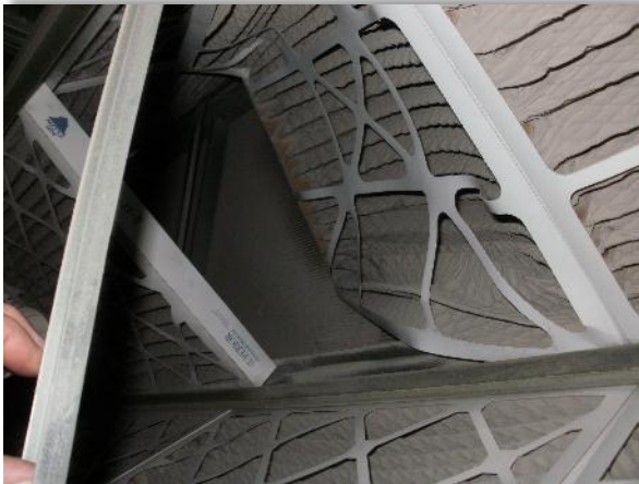
Filters plugged and pulled into AHU
