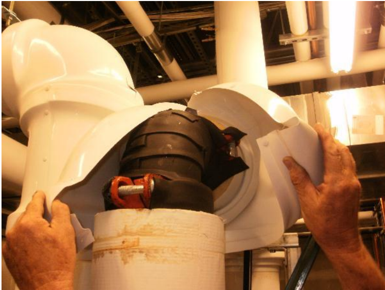
Incorrect insulation on fittings causing all fittings to drip condensation on floor
