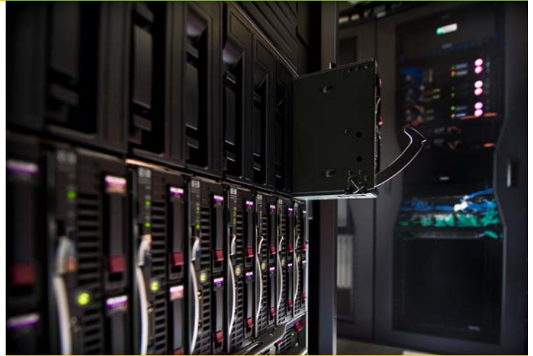
Figure 1. An example of RSF data center best practice implementation. Photo by Dennis Schroeder, NREL/PIX 18765
