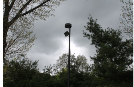
Pole-mounted lighting for unsheltered parking lots, including automobile dealerships
