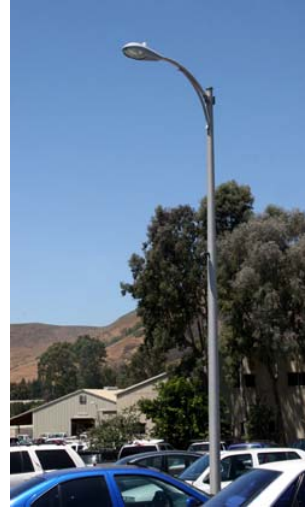
Bi-level cobrahead induction luminaire at California Polytechnic State University
