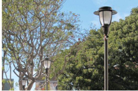
Bi-level LED post-top luminaire at the Los Angeles Trade Technical College
