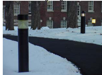
Bollards, luminaires used for path lighting, and which make their own architectural statement
