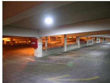
Bi-level LED parking garage luminaire at Sacramento State University
