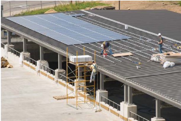
Solar - Photovoltaic Parking Garage, La Crosse
