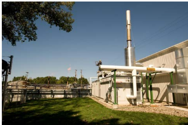
Biogas - Waste Water City Brewery, La Crosse
