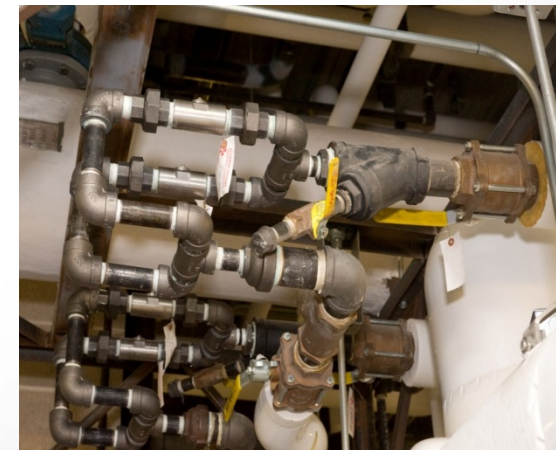
Insulation & steam traps
