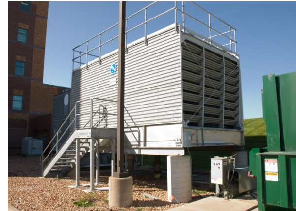
Cooling Tower Fans
