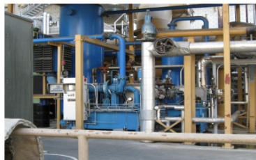
100 HP Steam Driven Air Compressor - Use of Let Down Steam Turbine (Tulare)
