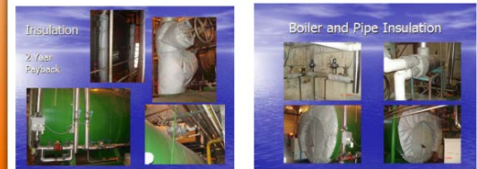
Insulation Blankets - Boiler Surfaces and Valves (Kiel)
