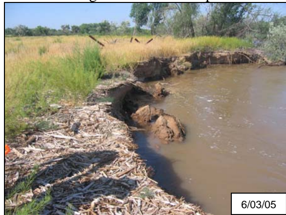
Figure 7: Small slump blocks fallen from the bank line at the bend apex on June 3 rd .
