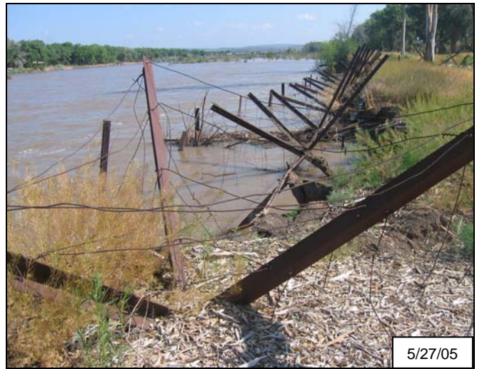
Figure 6: Bank erosion at the Priority Site on May 27 th , showing the erosion of sediments underneath the jetty jacks.
