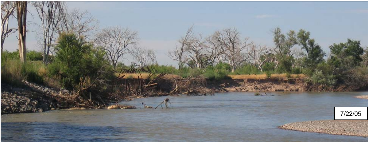
Figure 9: Site photo from July 22, 2005 that shows bank slumping along the bend apex, and a portion of the jetty jack line that has fallen into the river.
