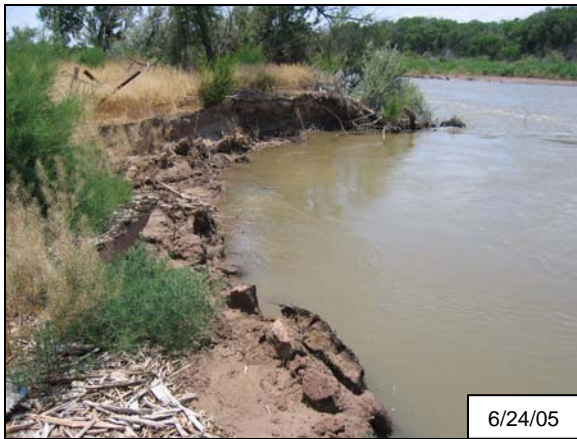
Figure 8: Extensive bank slumping/collapses at the bend apex; photo taken on June 24 th .
