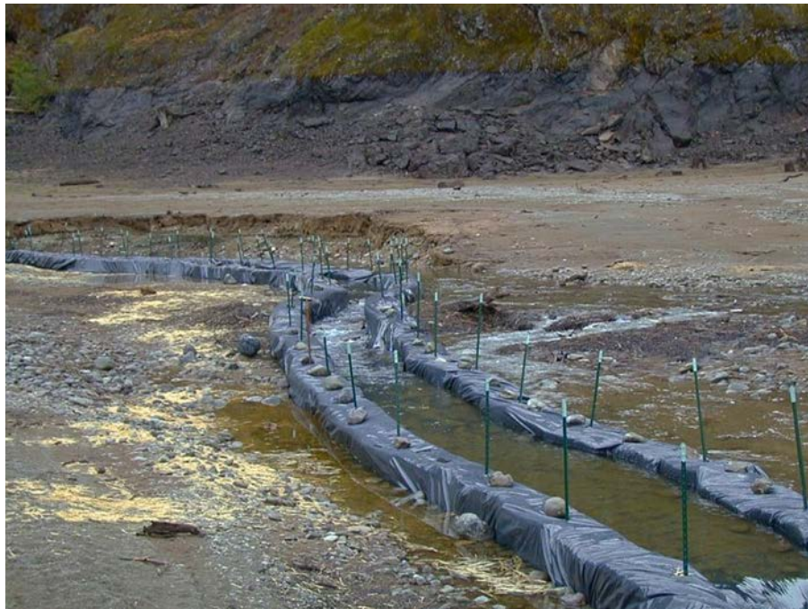
Figure 9-10. Box Canyon Creek temporary straw bale and visqueen passage channel for adult bull trout, 2003, looking up the creek as the flow is directed into the upper reservoir. It boosts flow depth in the cross-section and prevents creek flow from going subsurface before reaching the reservoir. Notice the bedrock outcrops along the canyon wall.
