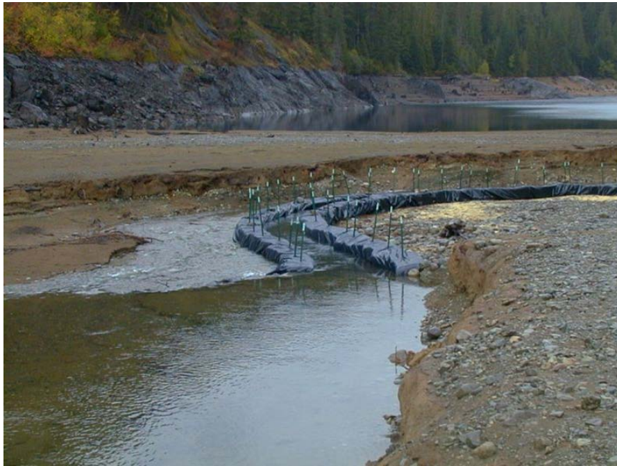
Figure 9-9. Box Creek Canyon temporary straw bale and visqueen passage channel for adult bull trout, 2003, looking downstream toward the upper reservoir. Built and removed four times in the past 14 years costing approximately $35,000 each time
