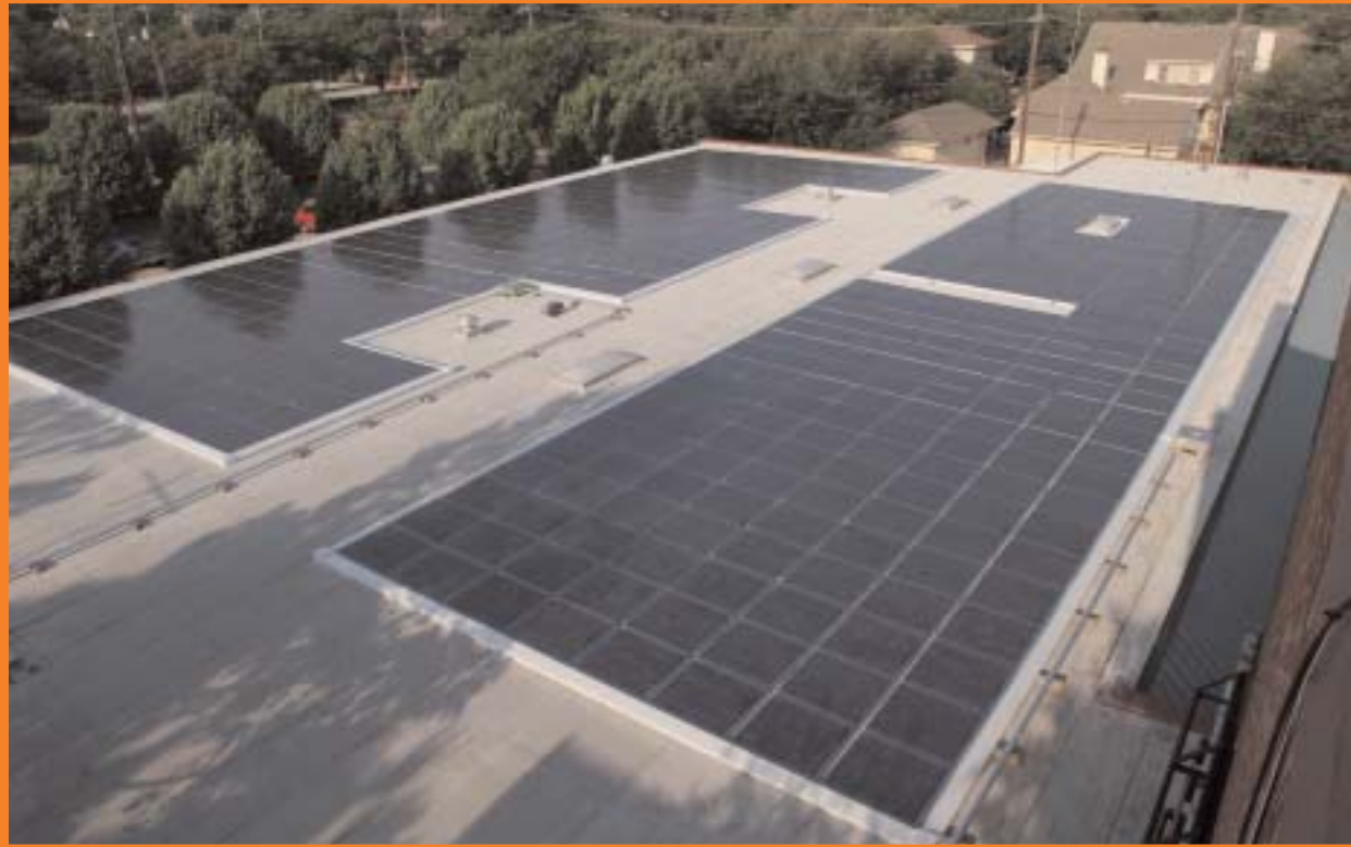
The Green Mountain Energy sm solar installation at The Winston School in Dallas, Texas, generates pollution-free, renewable electricity.
