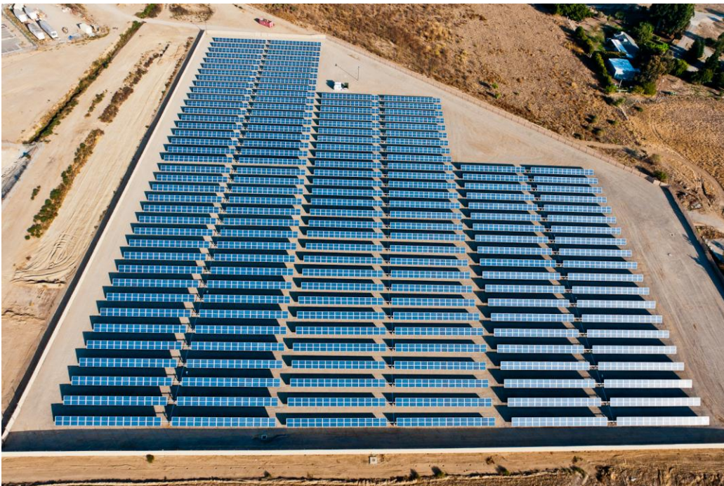
The 1.14 MW Madera Community Hospital ground-mounted array Photo credit: Borrego Solar
