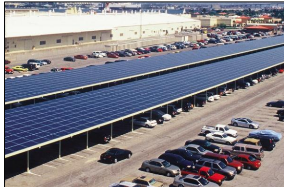
A large commercial carport-mounted PV array. Photo Credit: National Renewable Energy Laboratory.
