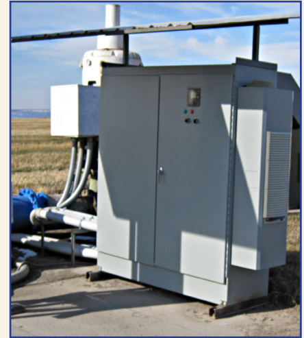
Housing for variable frequency drive
