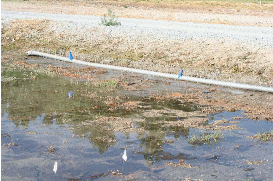
Perforated irrigation pipe watering the pond.
