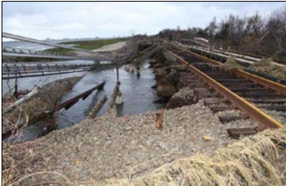
Damaged MTA A Train track at the Rockaways
