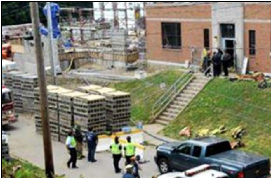
Elevated Facility Control Building
