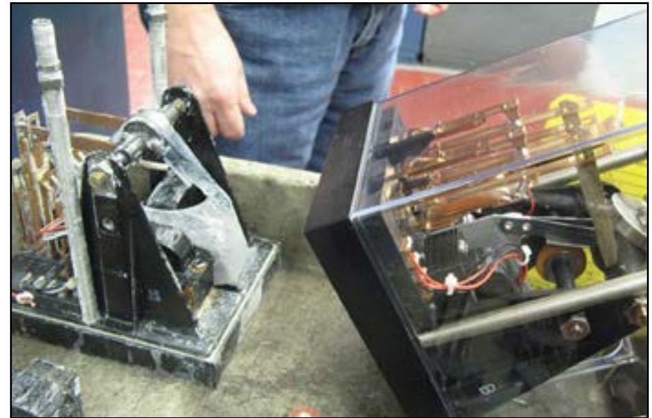
Storm-damaged and new Signal System Component
