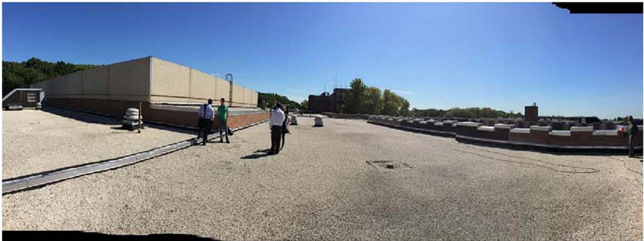
Figure 8. Roof of the Susan Wagner High School, looking south in Area 1 Photo by Kari Burman, NREL
