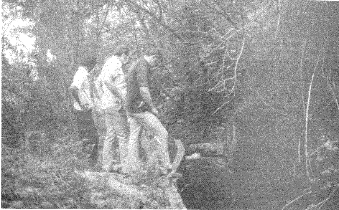
PHOTO NO. 2 - The Waimanalo Irrigation System ditch below the tunnel outlet on Aniani Nui Ridge.
