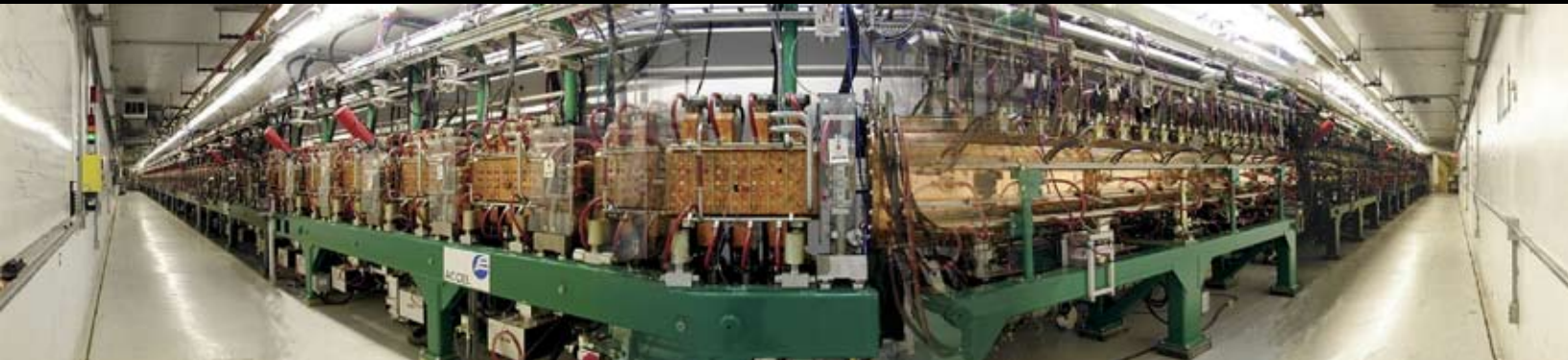
The Spallation Neutron Source, an extraordinarily complex facility, contains more than 100,000 control points.
