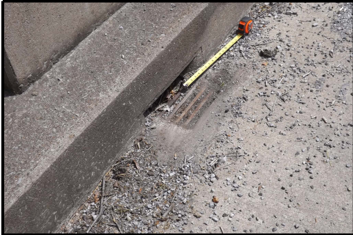
Gravel and debris along edge of deck plugging drain grate (typical of several areas)
