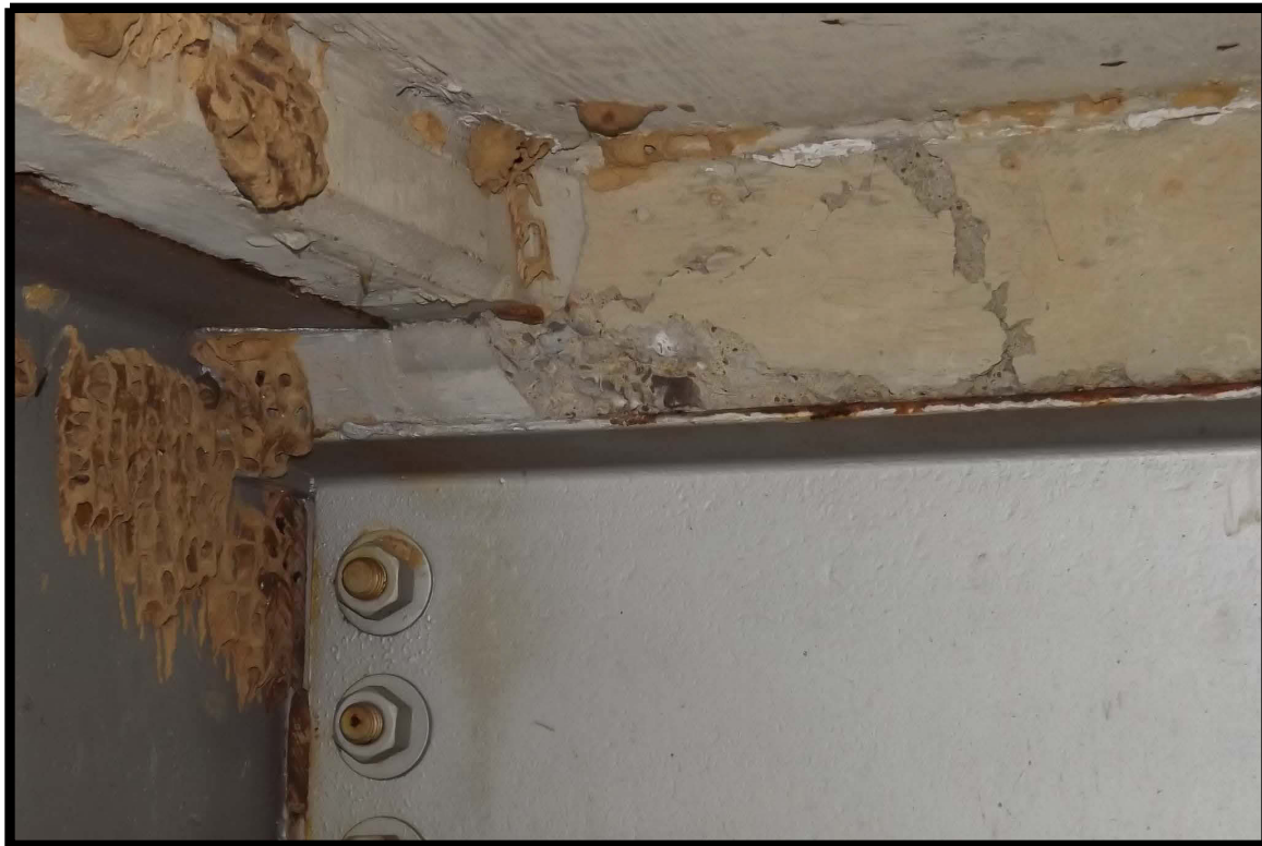
Cracks and spalls in haunch below deck at corner of diaphragm and girder at the abutment (common in similar corners of both abutments)
