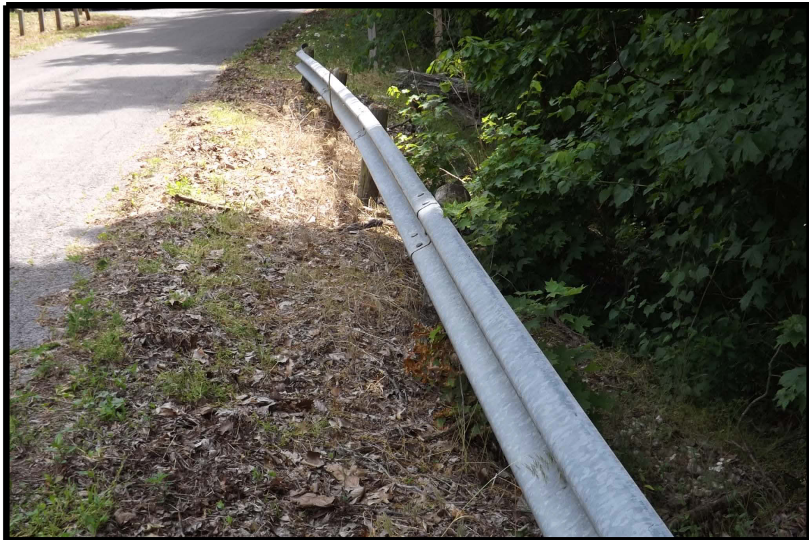
Southwest approach rail bowed and leaning away from roadway
