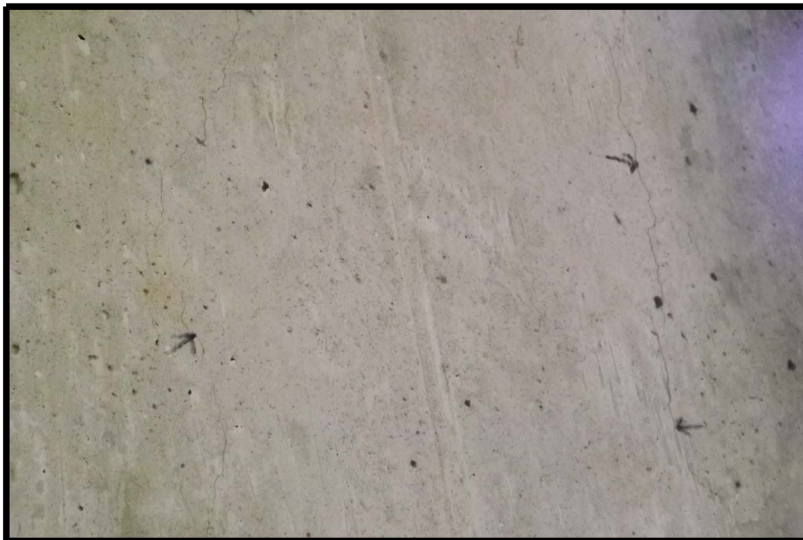
Close-up view: Fine vertical cracks (two are marked) on inside face of west column at 1st bent from south
