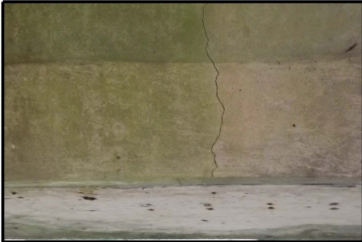
Tensional crack on lower 1/3rd of south face of 1st bent cap from south (largest of several between the bent columns)
