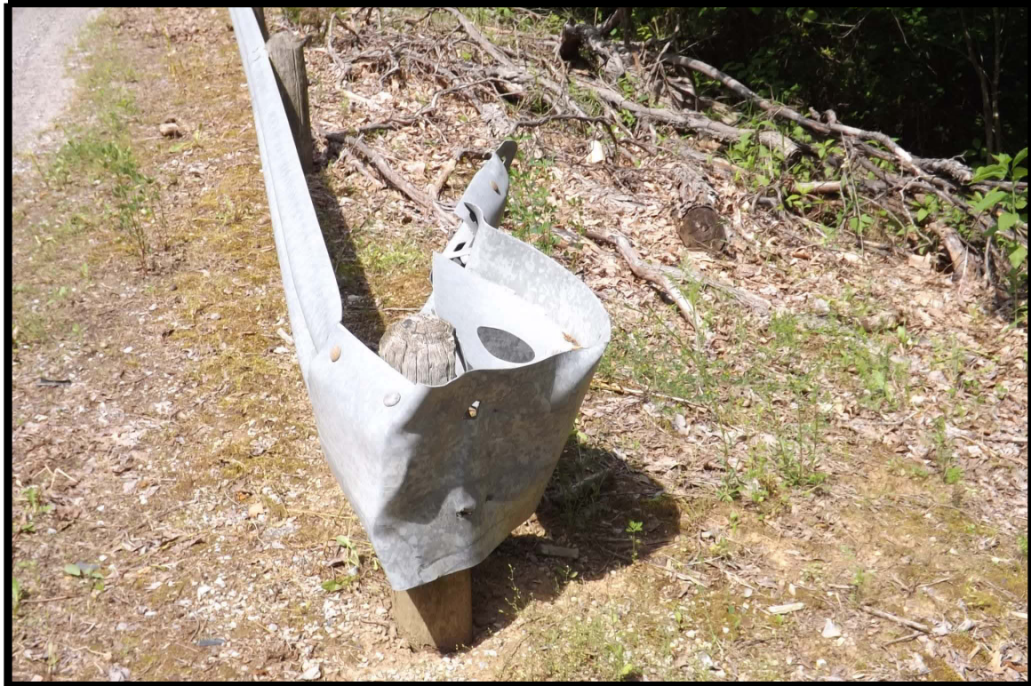
Impact damage to end treatment on southeast approach rail
