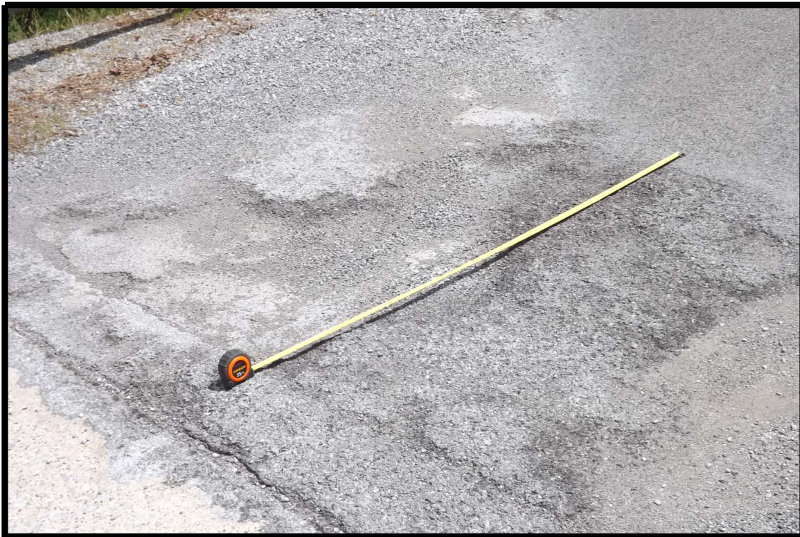
Large pothole in wheel path at south approach causing bump onto bridge (similar in other path)
