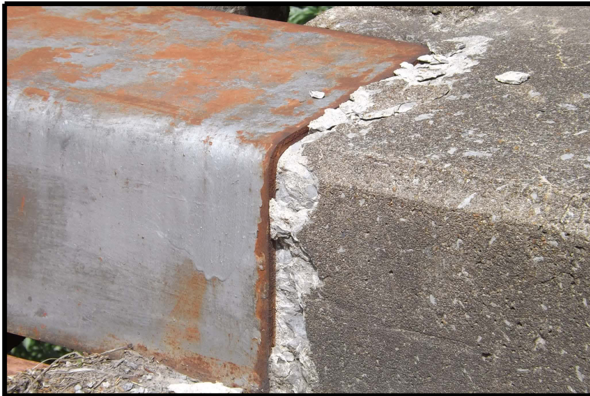
Damage to north end of east curb due to movement of expansion joint bridging plate
