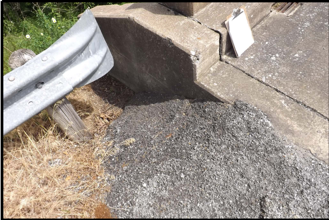
Prior area of sloughing and low shoulder at northeast corner has been filled and covered with pavement (similar at northeast)
