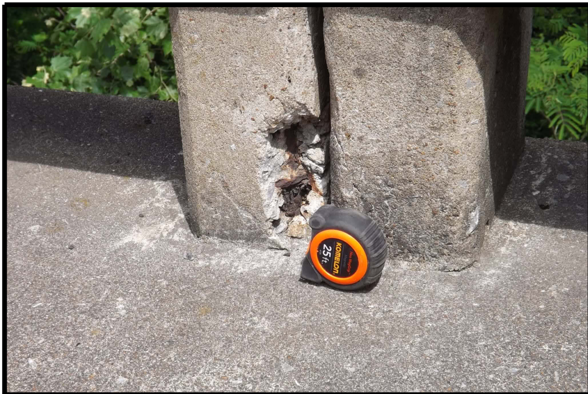
Spall with exposed reinforcing on lower portion of inside face of bridge rail post (typical of several)
