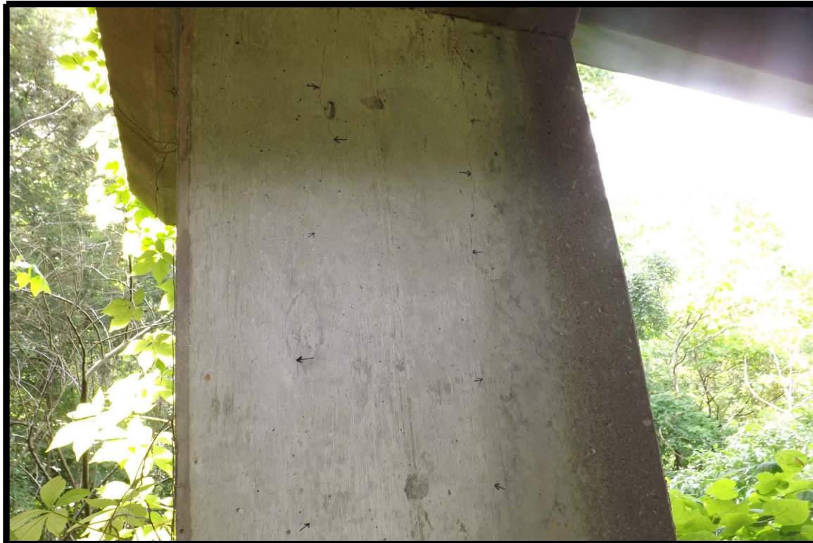
Fine vertical cracks (2-marked with arrows) on inside face of west column at 1st bent from south
