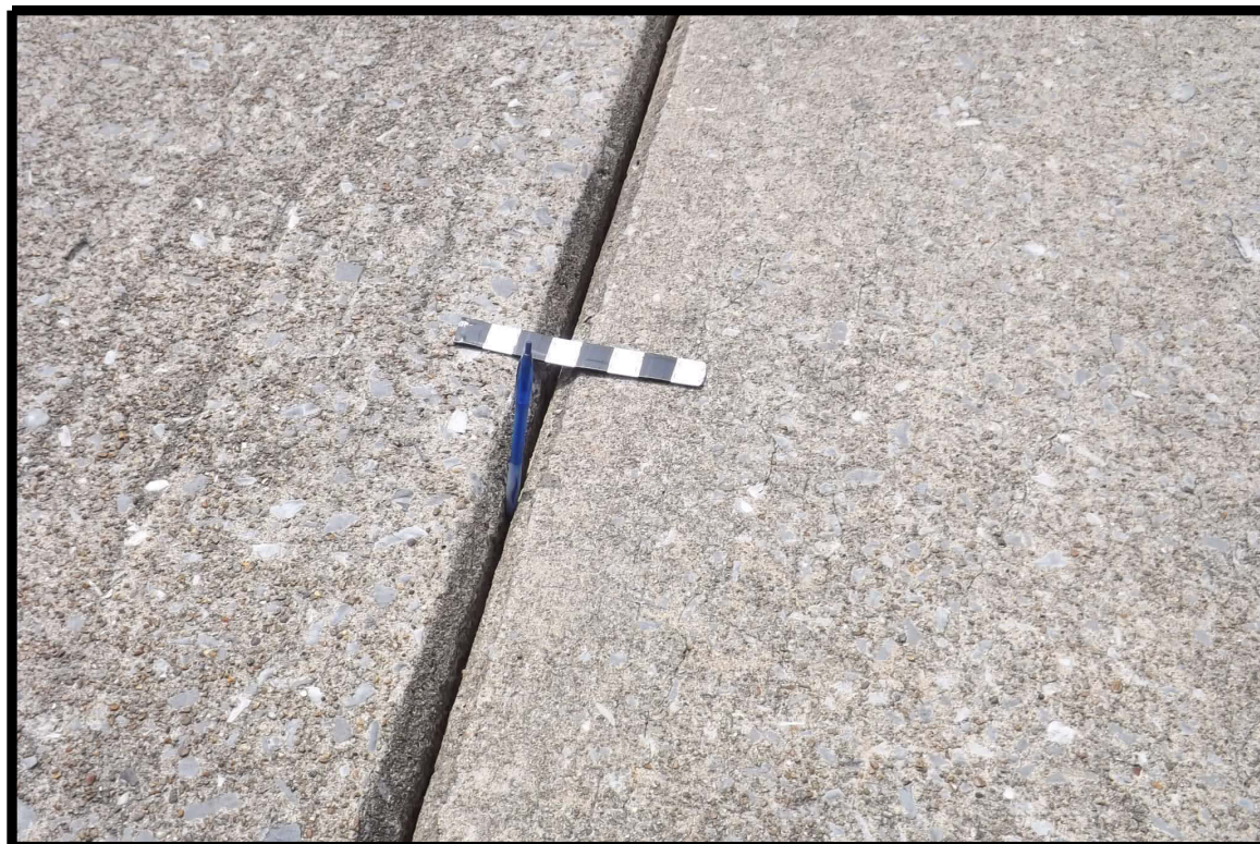
Open transverse joint in deck over 1st bent from north
