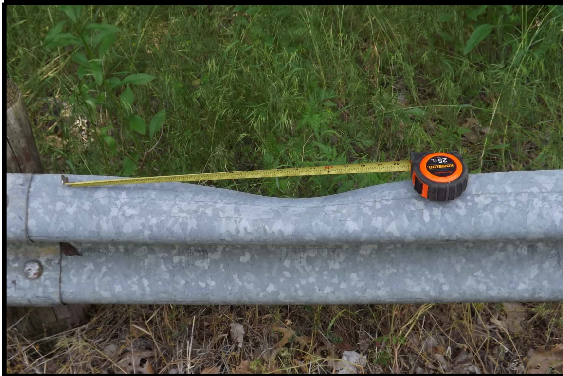
Damage, possibly from fallen tree, to top of southwest approach rail at the approximate southern 1/3rd-point
