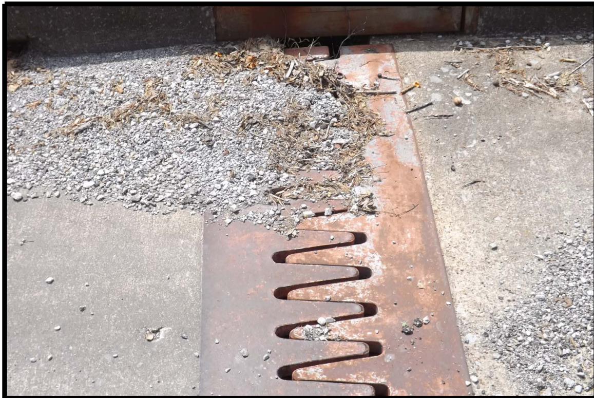
Gravel and debris at edge of bridge filling expansion joint opening (typical)
