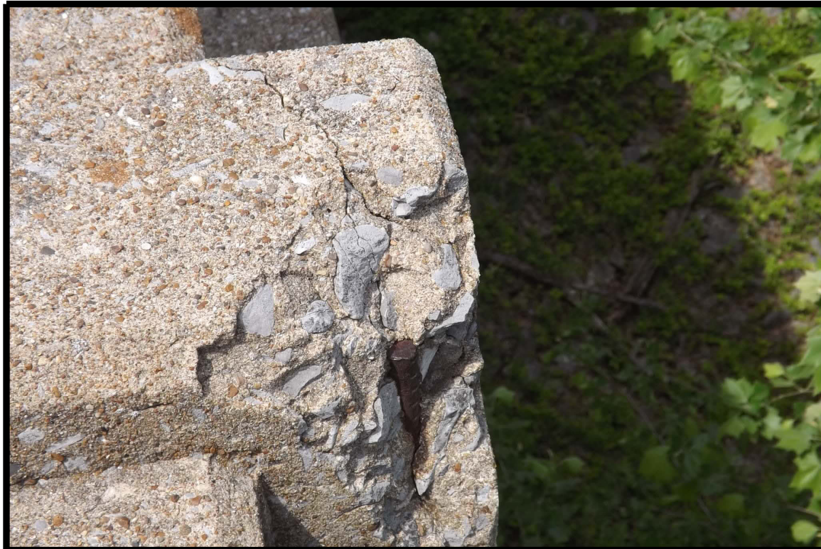
Crack and spall with reinforcing exposed on top and end of 15th bridge rail post from north on the east side
