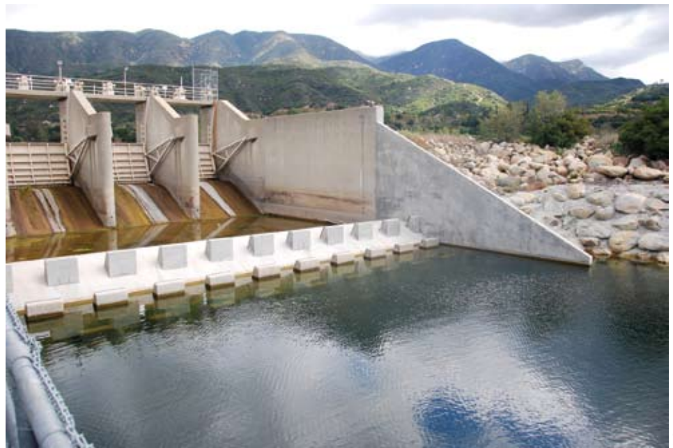
The Robles Diversion Dam and fish passage facilities on the mainstem Ventura River in early 2004.
