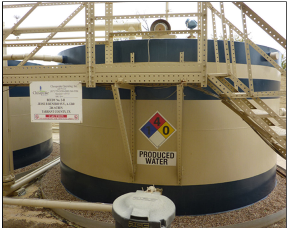
Figure 12: Storage Tank for Produced Water in the Barnett Shale
