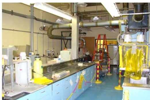
X-345 Laboratory Equipment for Strip-out
