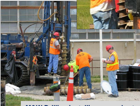
M&W Drilling installing groundwater monitoring wells. More than 1,000 monitoring wells have been installed at PORTS.
