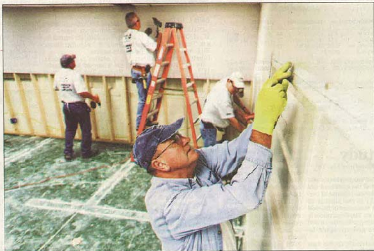
Dave Shrimpton, a risk manager for Fluor-B&W Portsmouth, prepares a window frame for new trim Friday at the Middleground Youth Center on East Water Street in Chillicothe. PHOTOS BY FRANK RODRIGUEZ/GAZETTE
